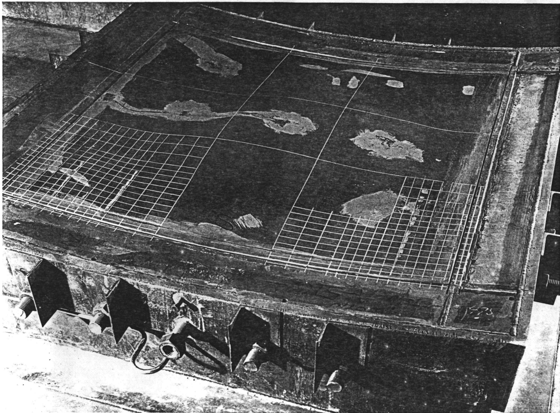
FIGURE 5. FT-3 Buckled Liner Plate.
