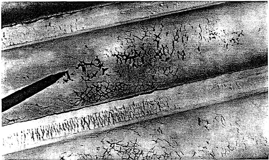
Fig. 7. Floor-tube panel from a North American boiler showing cracking in coextruded tubes. Cracks have been highlighted by dye-penetrant inspection. Cracks can be observed on the tube crown, at the tube-membrane interface, and in the membrane.
