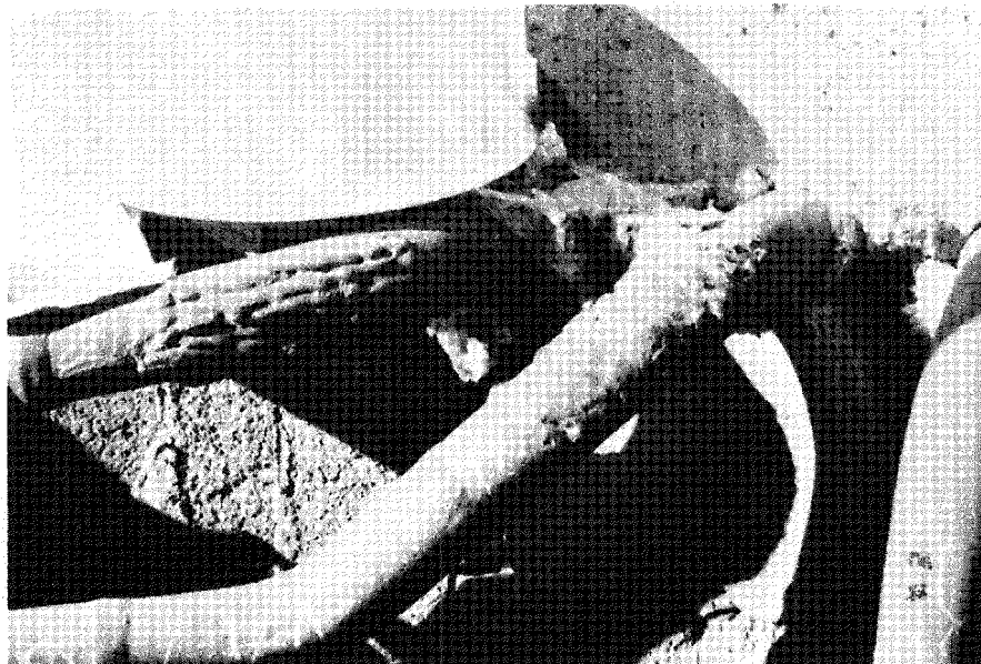
B-201-1B, GASIFIER SIDE FLOW HEATER-1, OCTOBER 20, 1973, SHOWING MORE WELD OVERLAYS ON OUTLET ELBOWS.
