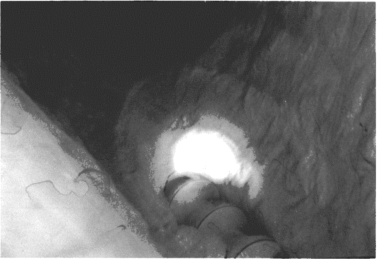
Figure 8. Ash Plugging ESP Field 1 Hopper
