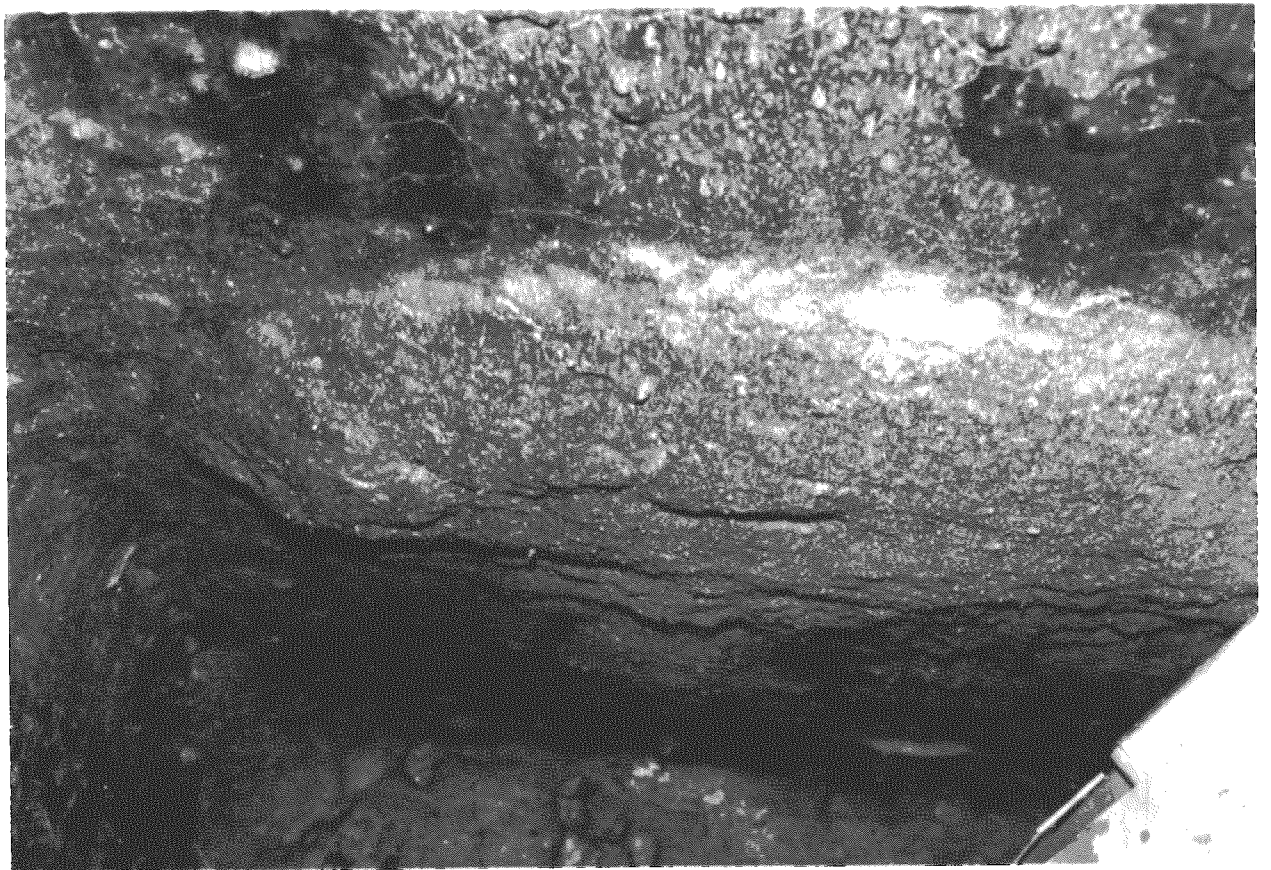
Figure 5. Primary Furnace Rear Wall Refractory
