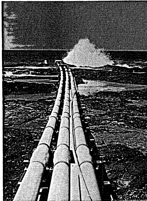
Waves break over cold and warm water pipes at NELH.
