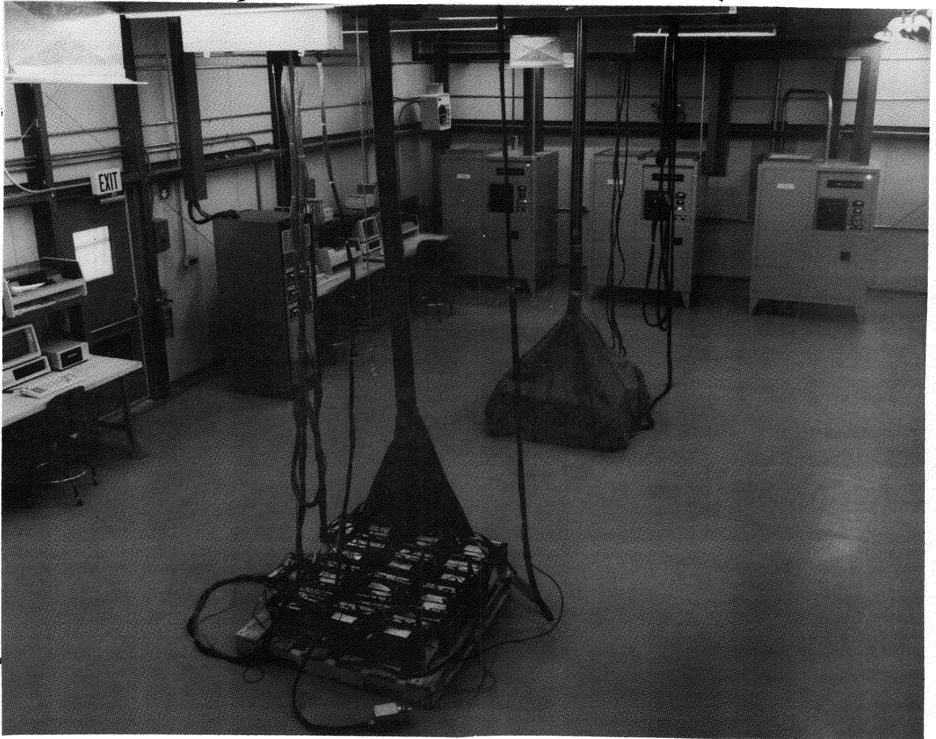
Figure 2. Photograph of the INEL Battery Test Laboratory
