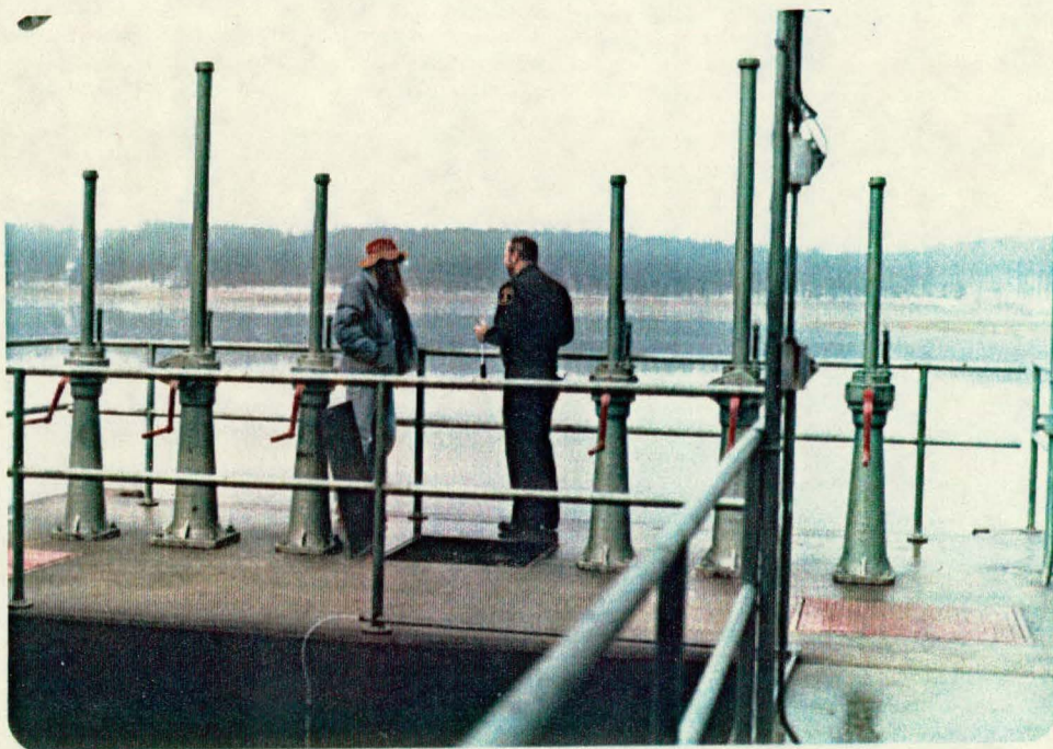
Intake Tower and Controls for Gates
