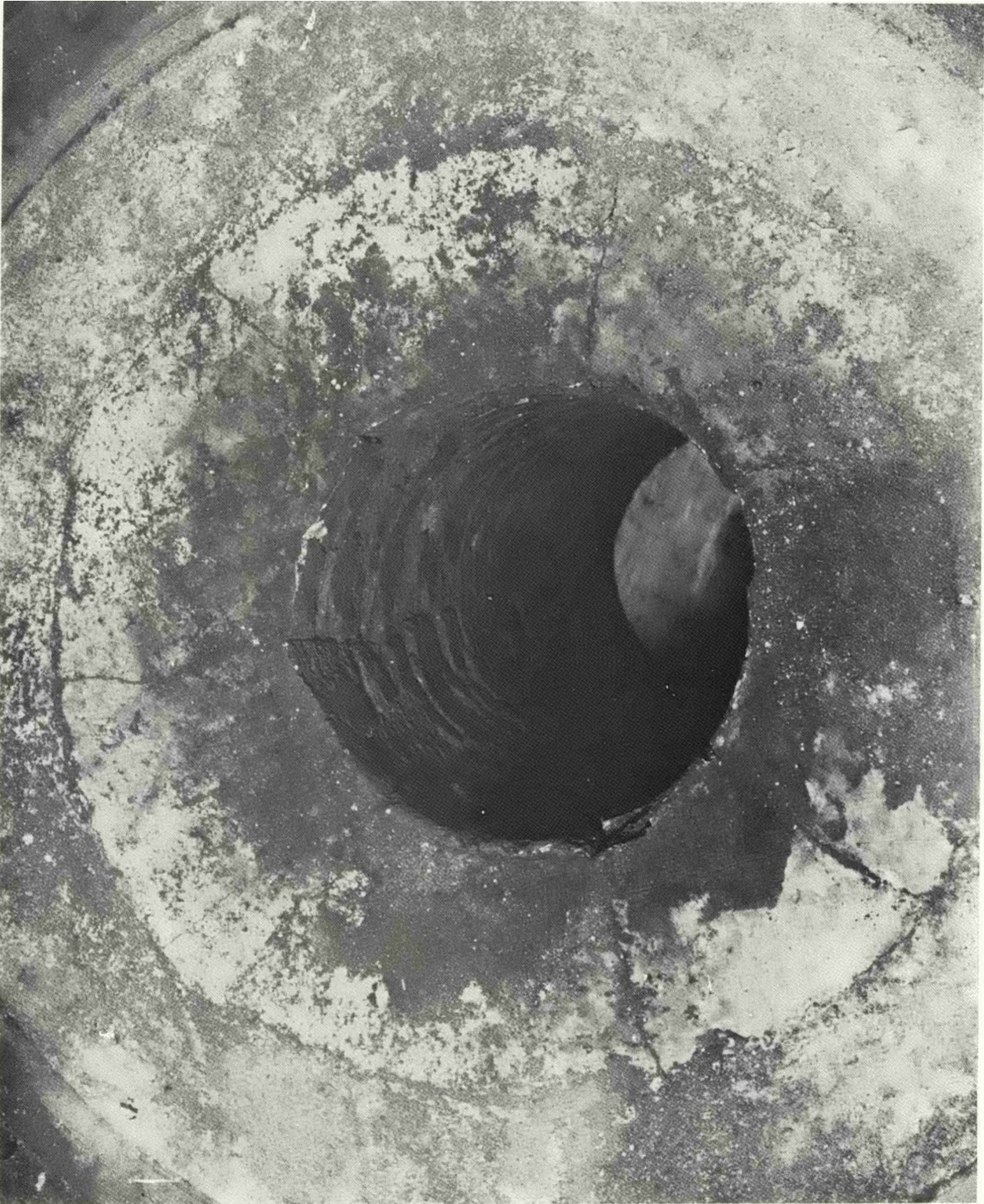
Figure 3.1-2. Gasifier Annulus Section Following Two and One-Half Years of Severe Operating Conditions with Over 40 Temperature Cycles. (Post-Test TP-019-3 Inspection)
