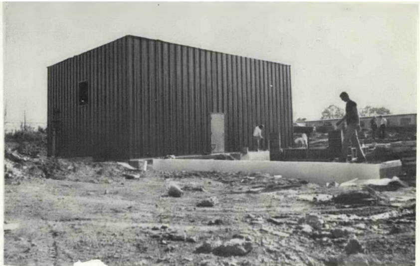
(Right) Compressor Building Shell Erected and Foundation Forms in Place for the Model Structure
