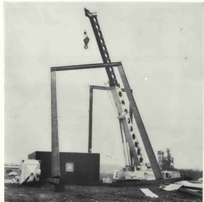
(Right) Erection of Model Structure Begins with Steel Framework which Dwarfs the Smaller Compressor Structure
