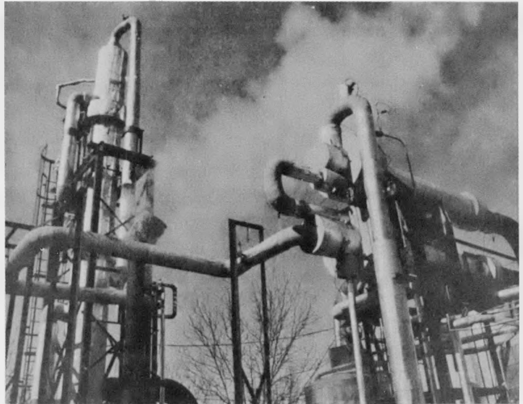
(b) Heat Exchangers; Condenser/Evaporator at Left, Superheater/Désuperheater at Right
