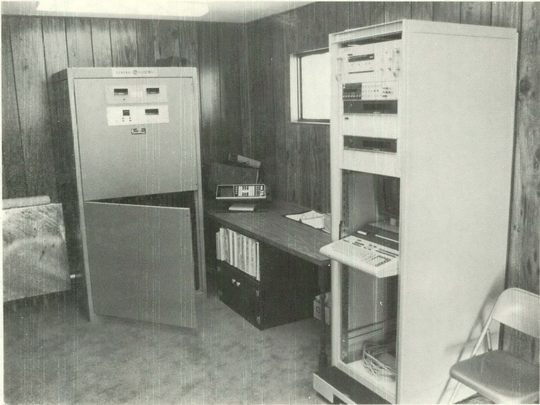
Figure 11. ODAS and DC Switchboard in Visitor Center
