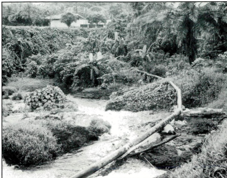
(Penstock for transporting water to the turbine - PICS - 1982.)
