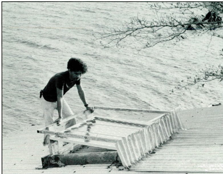
(Photovoltaic array on the roof of Micronesia Bound - 1983.)
