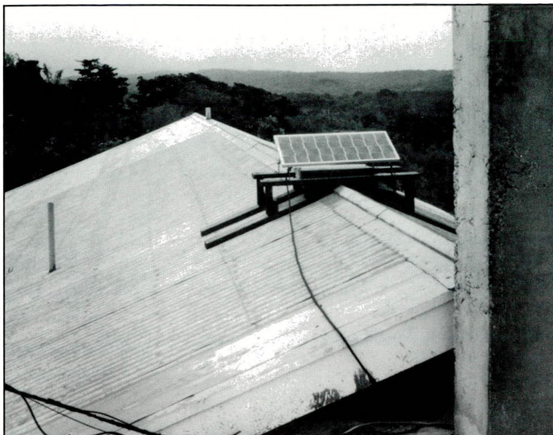
(Part of the photovoltaic refrigeration system at Aimeliik Elementary School, Palau - 1985.)
