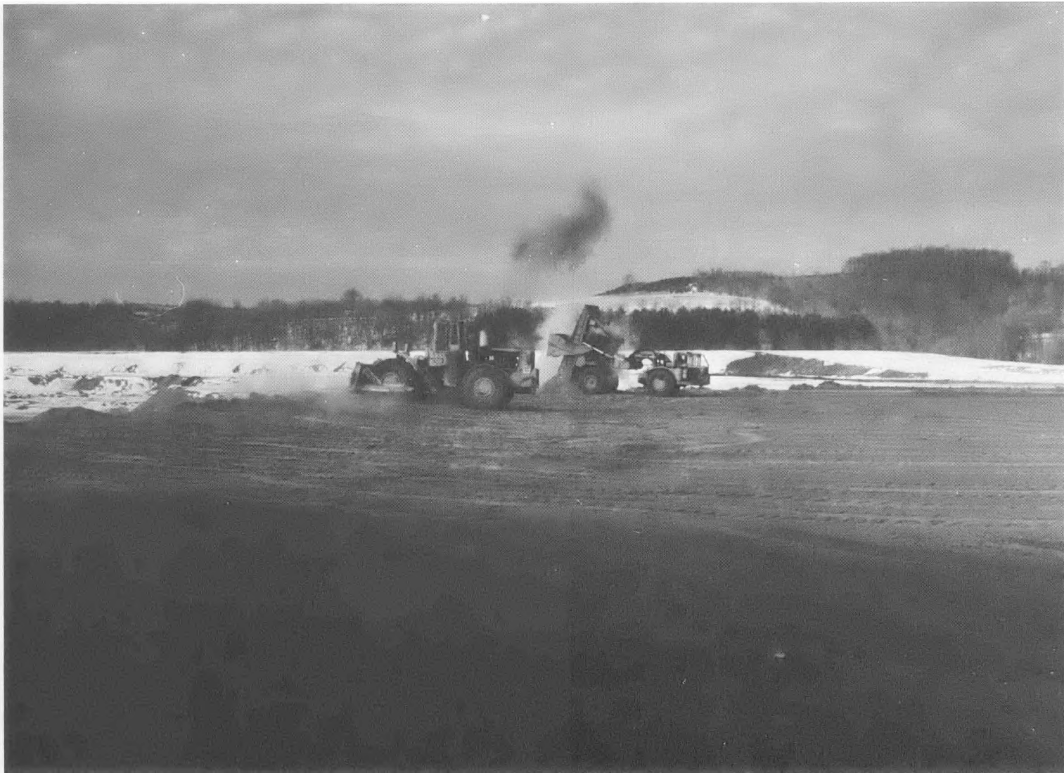
Figure 6-14. Ash Placement, Keystone Station
