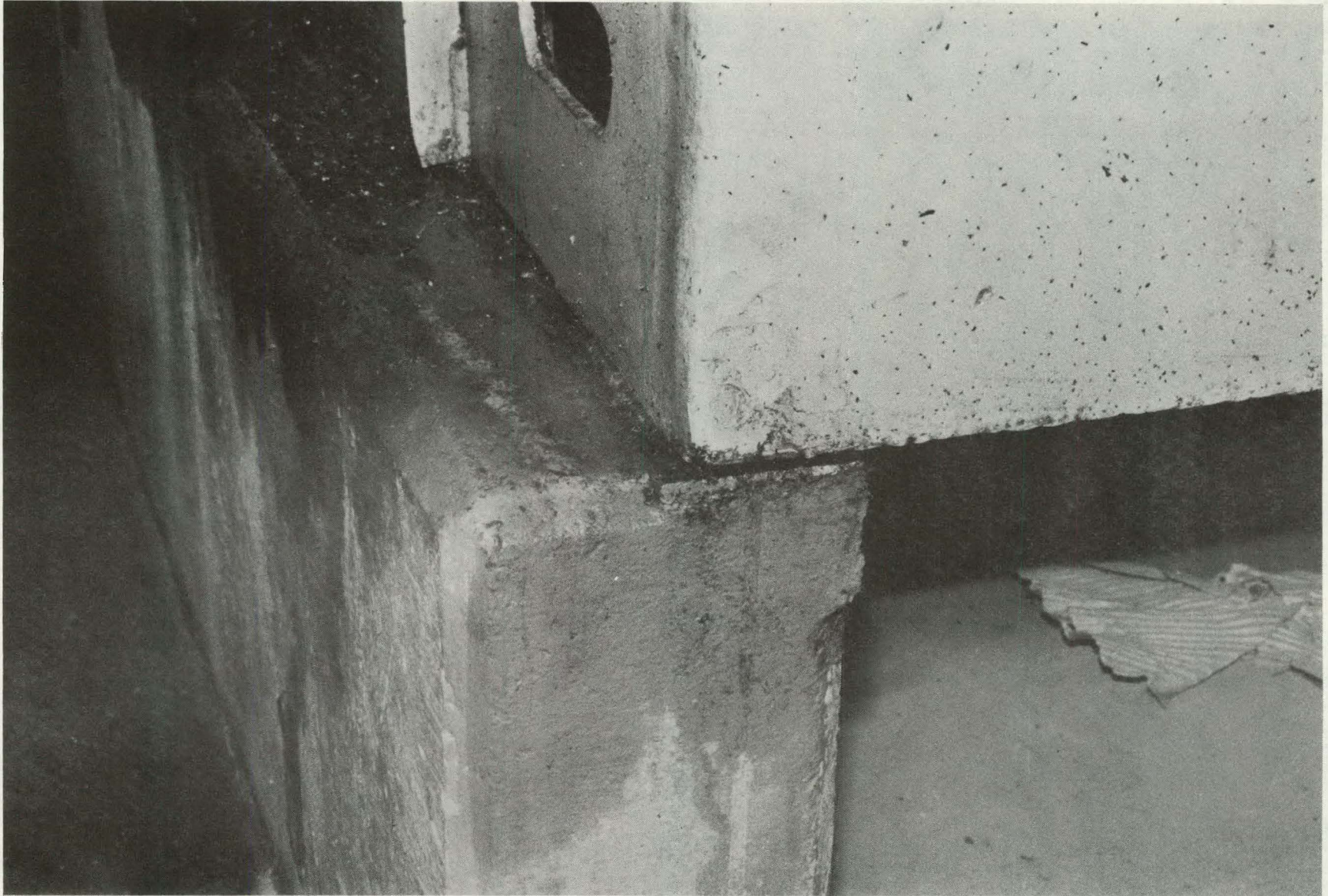
6 Turbine oil cooler tank anchorage
