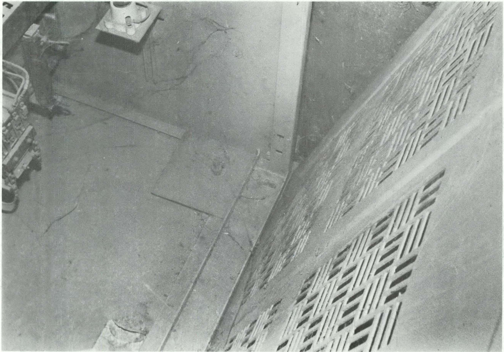
8 Exciter cubicle anchorage
