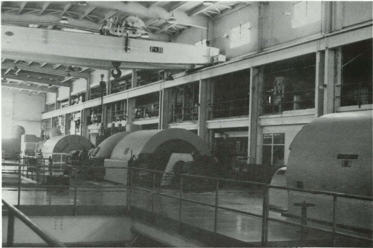
Fig. 17. View, looking south along the row of turbine-generators toward Unit 4, shows that there are no E-W partitions between the structurally separate units.
