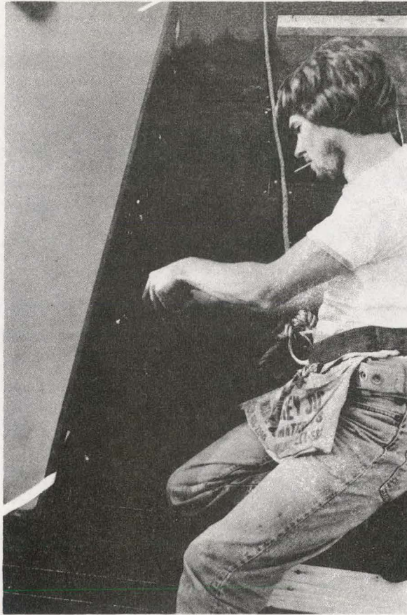
Figure 2-13. Collectors Secured to the Roof with Lag Bolts
