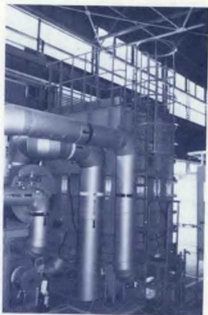
Figure 3. 10kW class test facility
