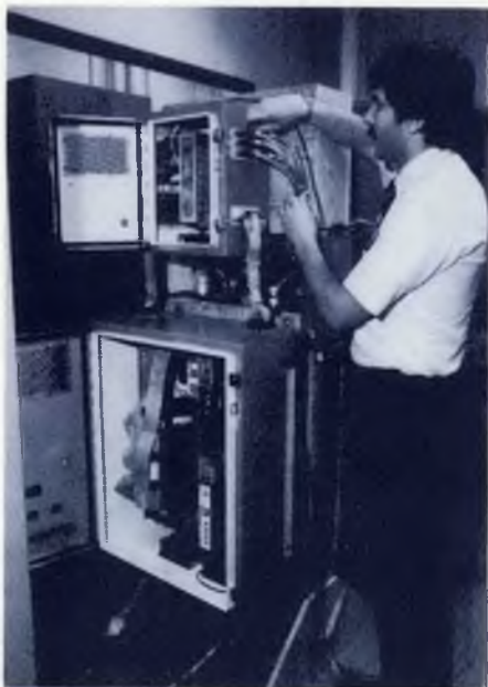
Figure 4. Control Unit for Power Switching Pole Test
