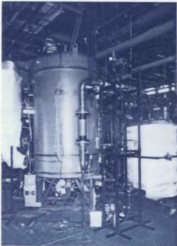
Figure 2. FUEL PROCESSOR - INSTALLATION IN TEST STAND
