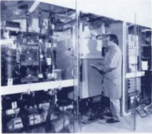
FIGURE 3 5 KW GENERATOR AND TEST FACILITY
