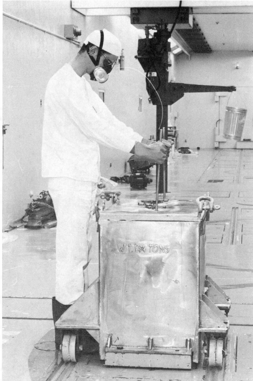
FIGURE 22: Filter Disposal Flask in Position to receive Ventilation Filters
