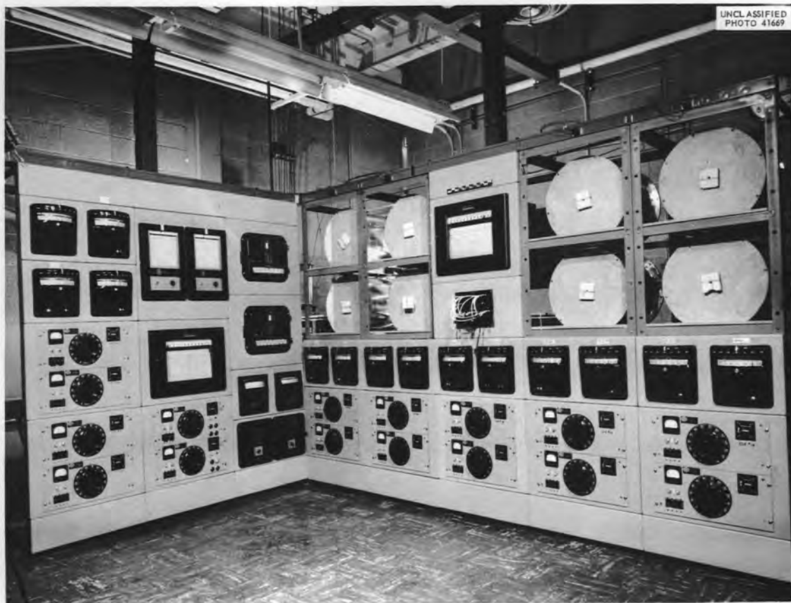
Fig. 42. Furnace Control Panel, Metallurgy Laboratory.
