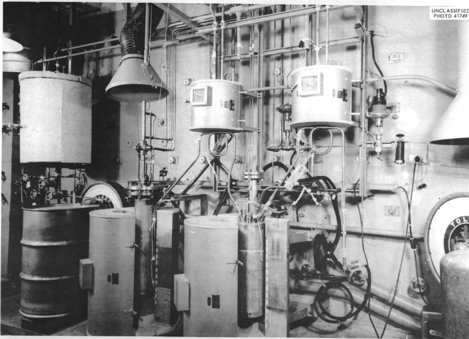
Fig. 21. Laboratory-Scale Hydrofluorination Facility for Power Reactor Fuel Element Dissolution.
