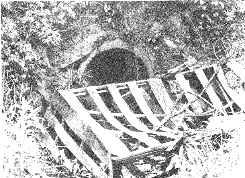
Figure 22. Trash in creek in Sub-basin W-2.
