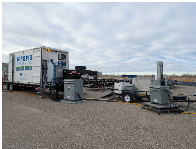
Fig. 4. An image of the MIB class microgrid used in the experiments in this work is shown here. Some of the components visible outside the container are breaker panels, inverters (white), transformers (gray), and HVAC for the microgrid, while the rest of the components reside inside the container. The component list for the microgrid is shown in Table I.
