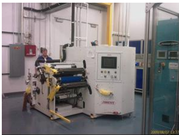
Figure III-31: New anode slitting station.
