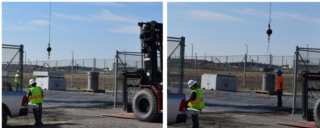
Figure 15. Removal of the ISC lid (left) and removal of the overpack cap (right).
