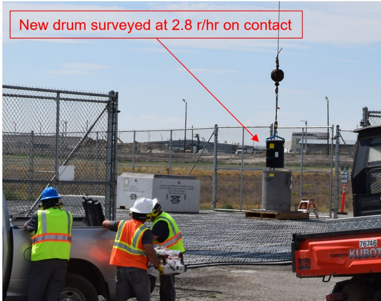
Figure 16. Lifting of the new 50-gallon waste drum out of the overpack with the crane.
