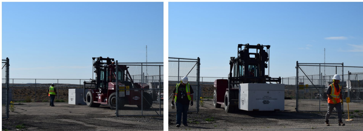
Figure 13. Lifting of ISC-007 with a forklift (left) and removal of the ISC from the storage area (right).
