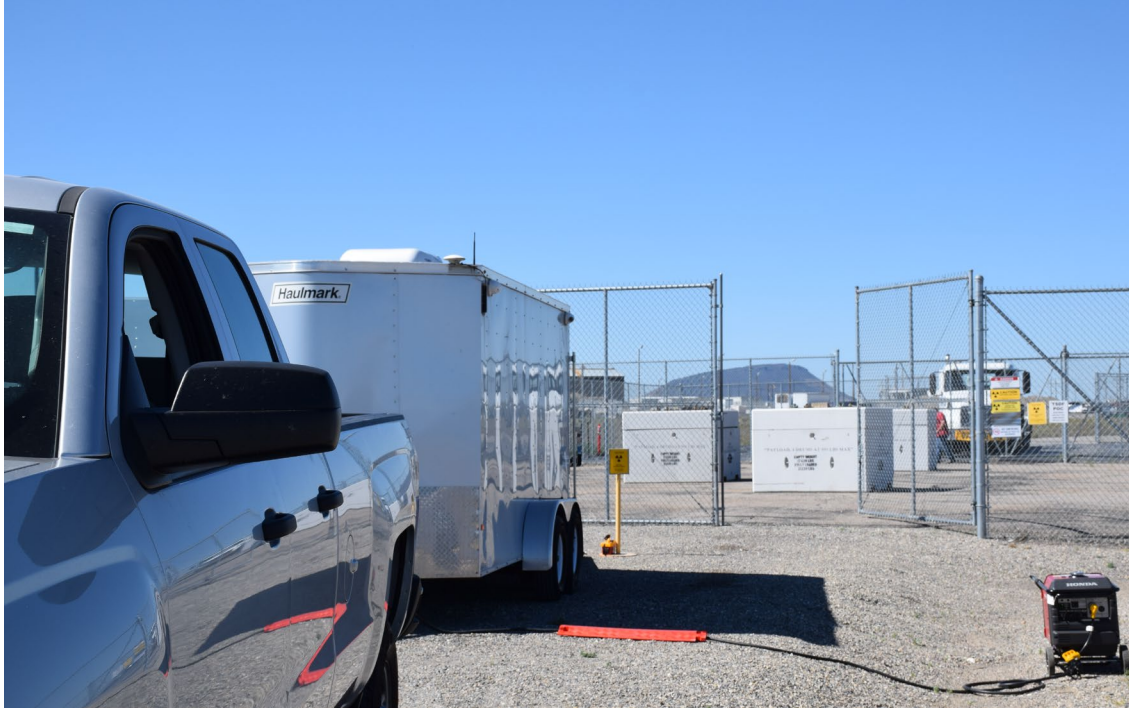
Figure 4. Field testing trailer with external generator to provide power.
