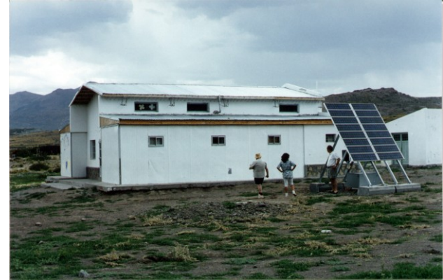
PV system with battery storage at a school in Colipar Abajo, Argentina. This system represents the type of microgrid configurations currently supported under the Microgrid Services Tariff. Photo by NLR
