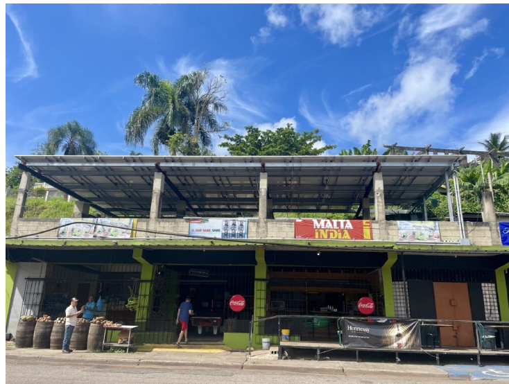
June 12, 2025 - In the rural community of Castañer, Lares, a small market building stands with solar panels mounted on its rooftop. This setup is part of a community microgrid project that provides renewable electricity to local residents. Photo by Glorynel Ojeda Matos, NLR
