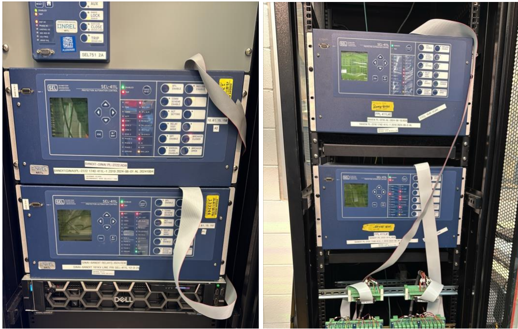
Figure 18. CHIL setup of SEL relays. Photos by National Laboratory of the Rockies
