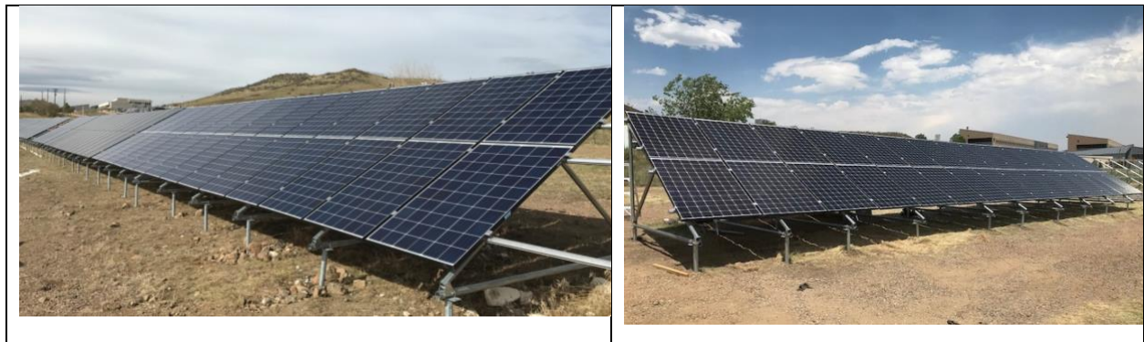
Figure 5. NLR PV Lifetime installations. QCells (left) and Panasonic (right)
