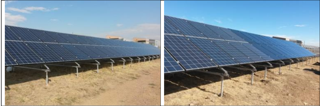
Figure 2. NLR PV Lifetime installations. Jinko Solar (left) and Trina Solar (right)
