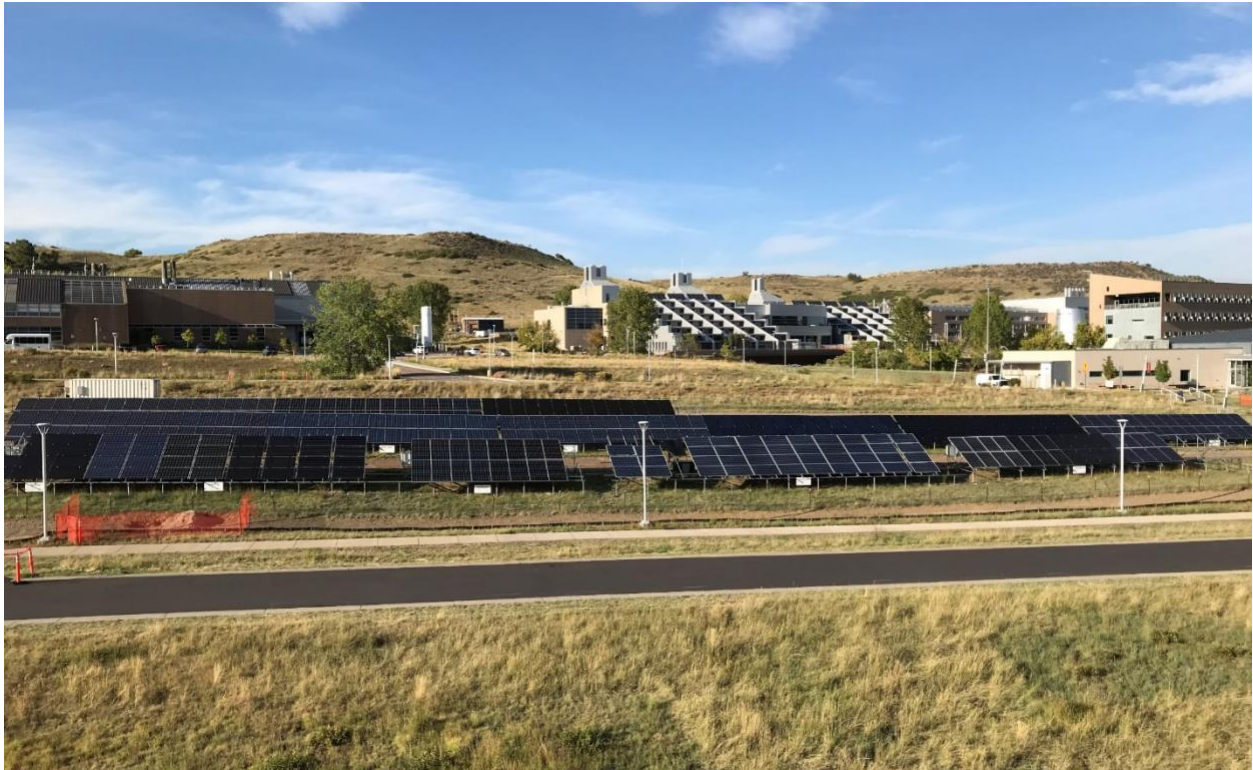
Figure 1. Overview of the NLR PV Lifetime field samples ca 2018
