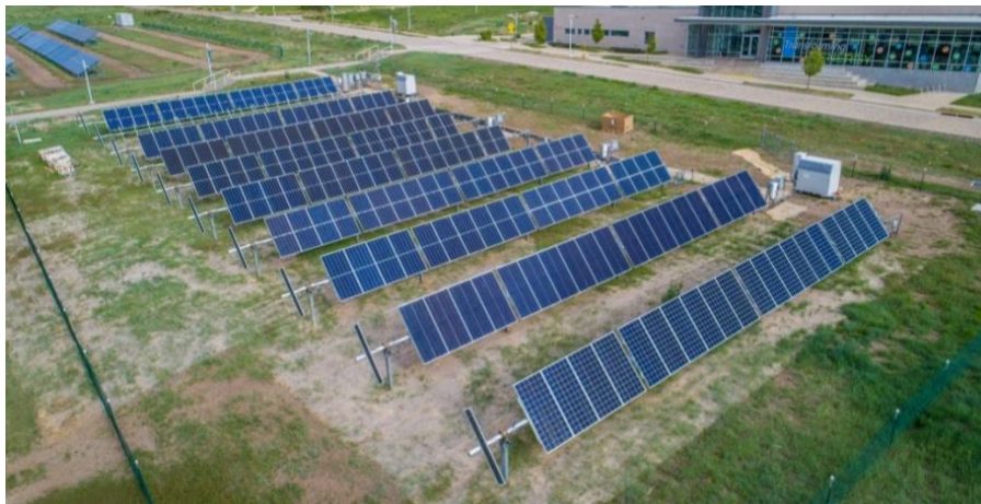
Figure 8. NLR 75-kW tracking PV system supporting PV Lifetime performance data
