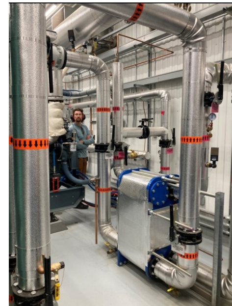
Heat exchanger. Photo courtesy of the Alaska Native Tribal Health Consortium
