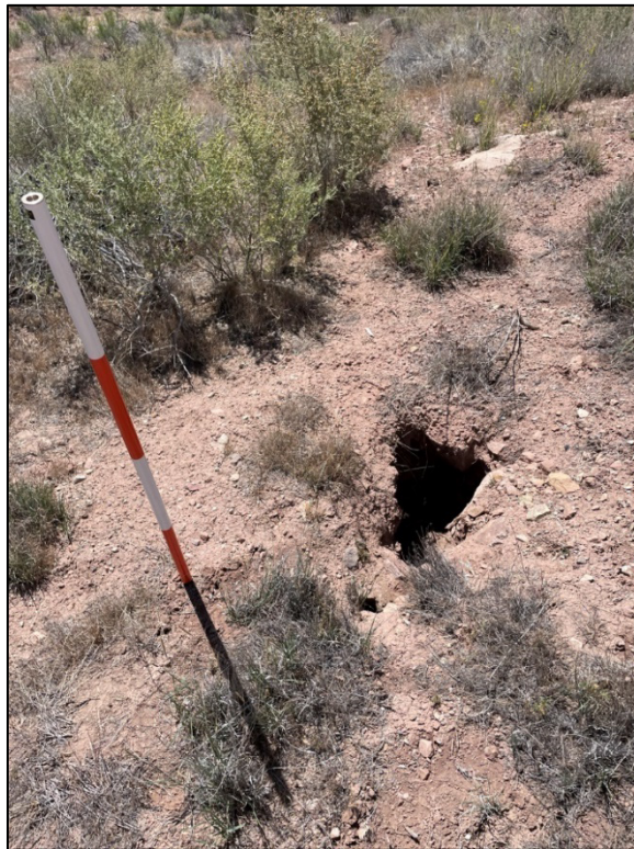
PL-8. Soil Piping West of Access Road
