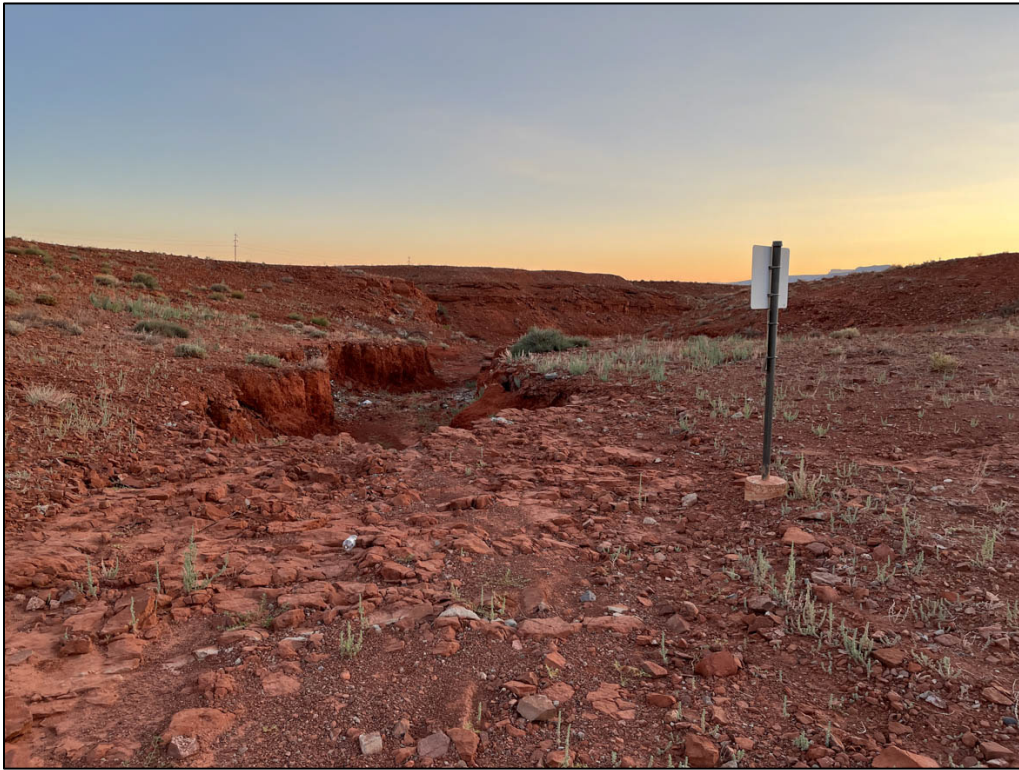
PL-13. Headcutting Encroaching on Perimeter Sign P43
