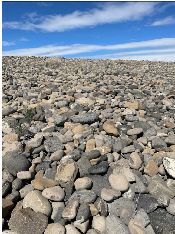
PL-8. Soil Infilling in Riprap Along East Side Slope
