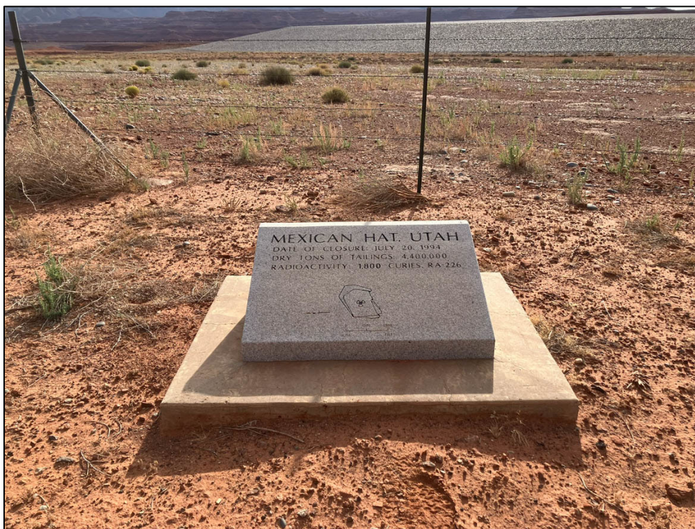
PL-7. Site Marker SMK-1 with Minor Cracks in Concrete Base
