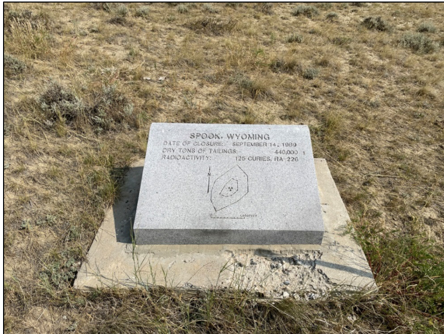
PL-2. Spalling on Base of Site Marker SMK-1
