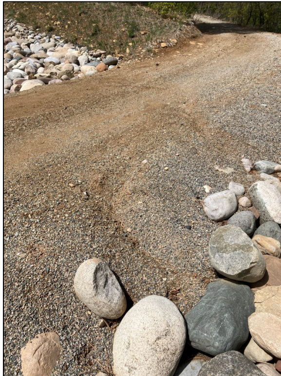
PL-1. Access Road Erosion
