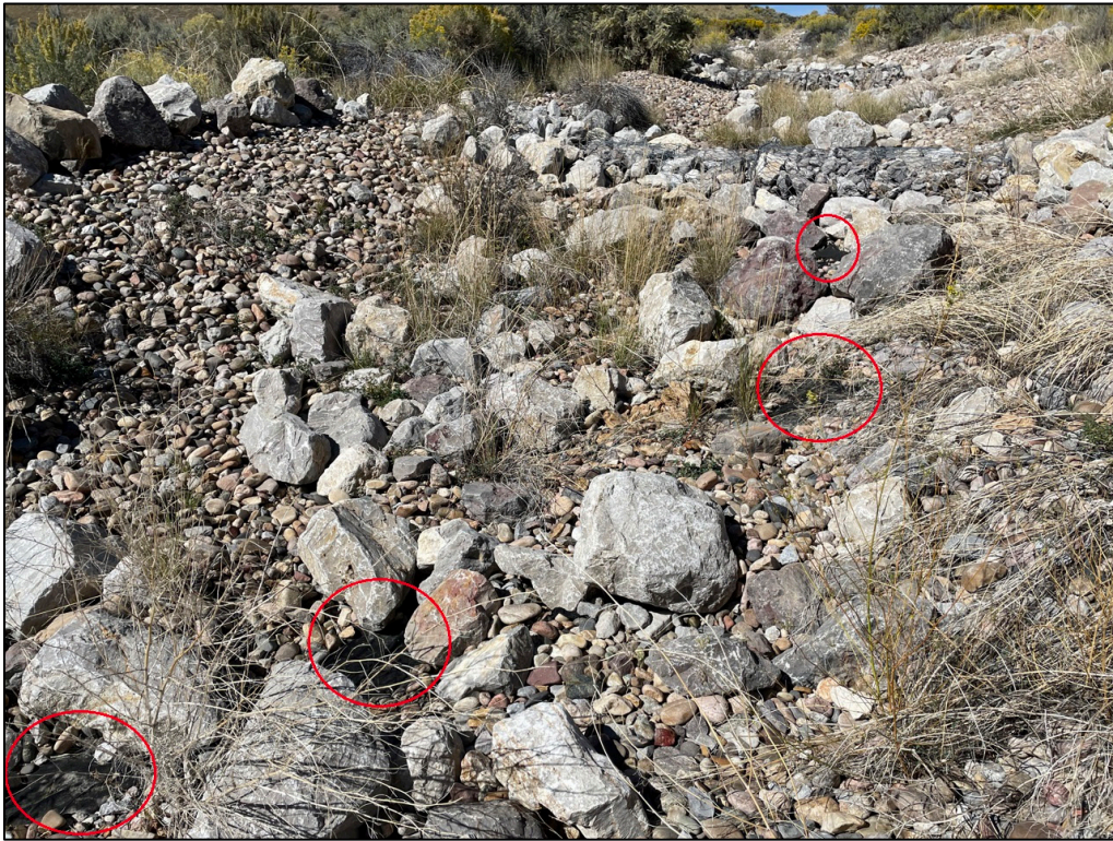
PL-7. Geofabric Exposed in Channel
