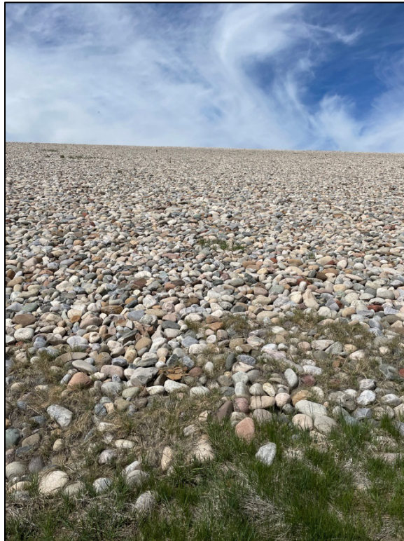
PL-11. East Side Slope—Sediment Accumulation and Vegetation Growth
