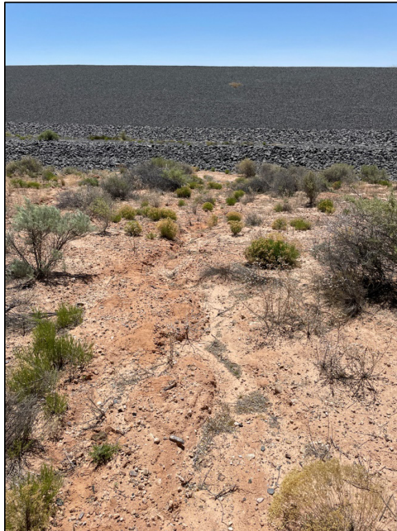
PL-13. Erosional Gully and Soil Accumulation in Diversion Ditch North of Disposal Cell
