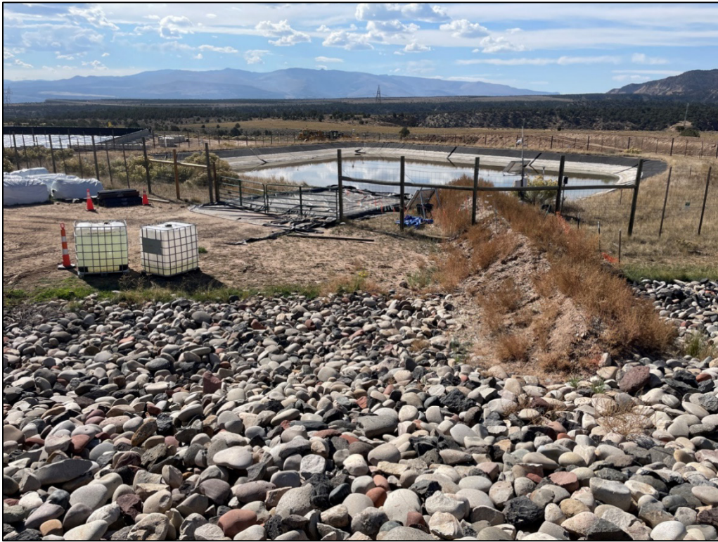
PL-5. Buried Discharge Line for Standpipes MW02 and MW03
