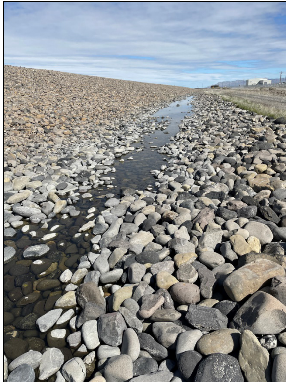
PL-10. Standing Water in Toe Drain near Southeast Corner of the Disposal Cell
