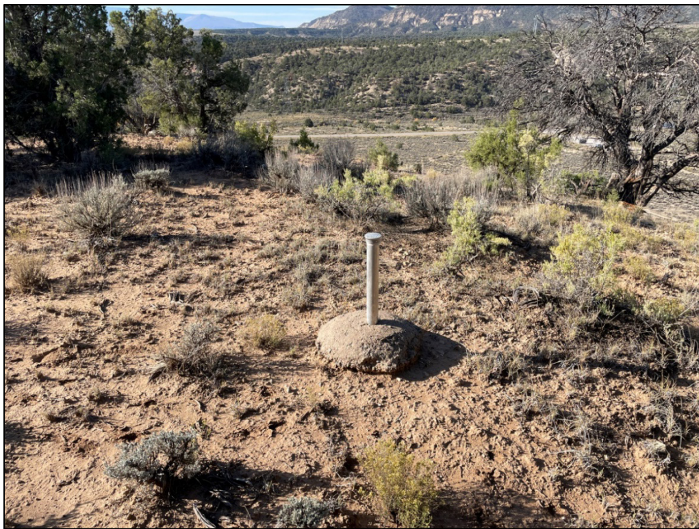
PL-4. Boundary Monument BM-16 with Undercutting
