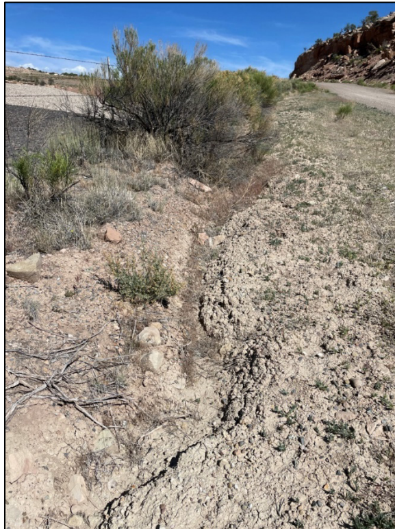
PL-9. Gully near Southeast Fence Line
