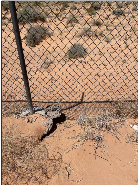
PL-1. Gap Under Fence near Perimeter Sign P9
