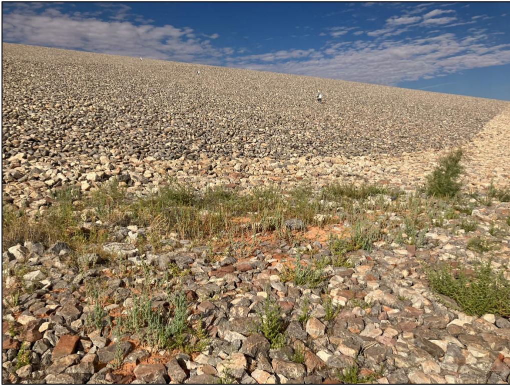
PL-11. Sediment and Vegetation Accumulation in Northeast Toe Drain
