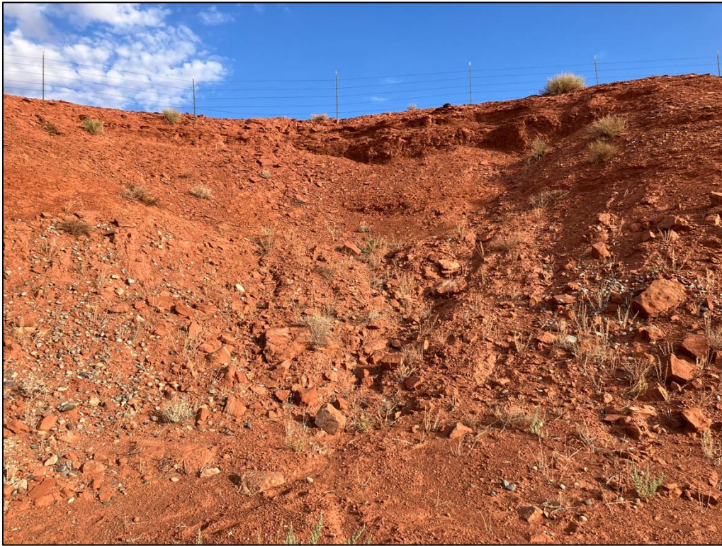
PL-3. Erosion Under Fence; Concrete Base Exposed
