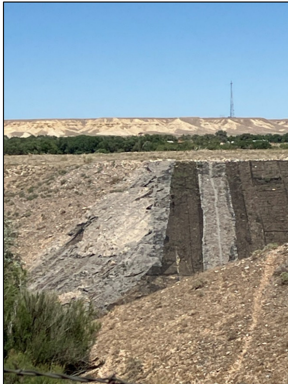
PL-13. Deteriorated Fabric in Outflow Channel
