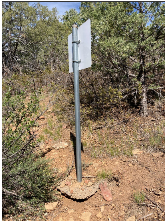
PL-6. Perimeter Sign P62 with Undercut Base and Unstable
