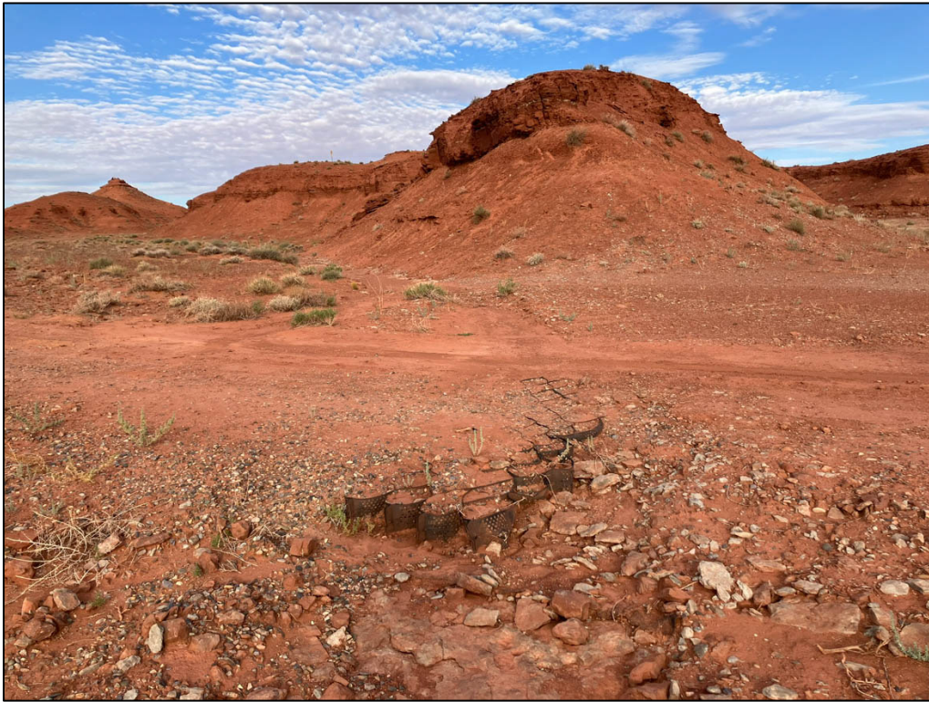
PL-1. Minor Road Erosion at Armored Drainage; Geocell Exposed
