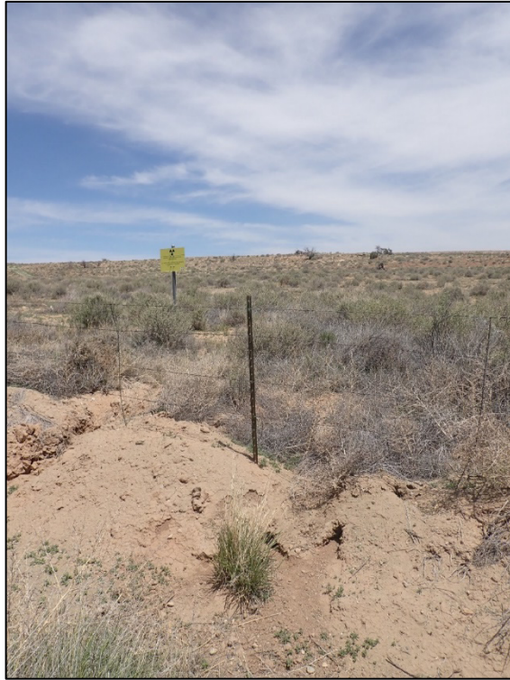
PL-3. Erosion at Fence Line Between Perimeter Signs P31 and P32
