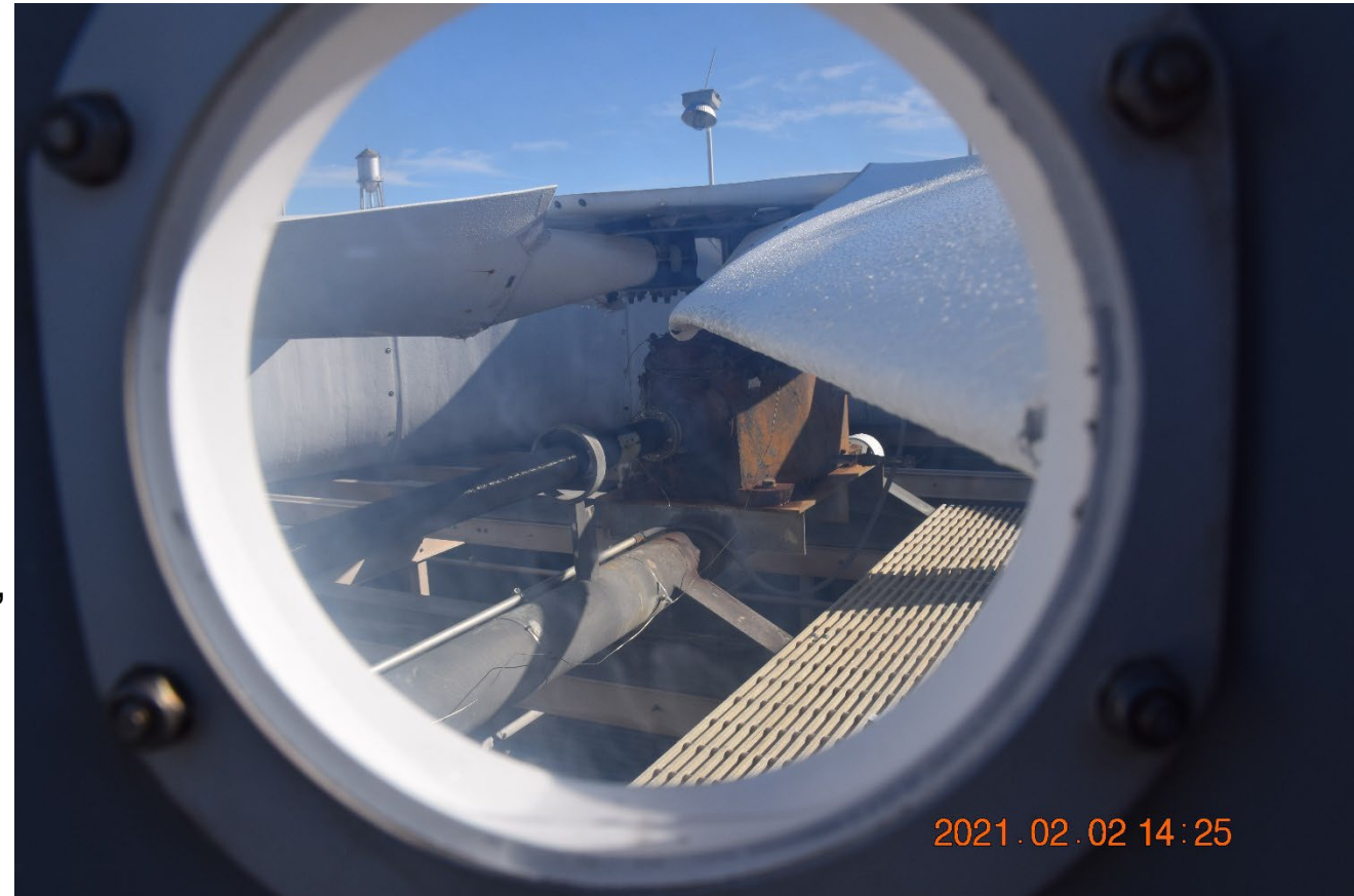
View of the gear reduction box for ATR fan #2
