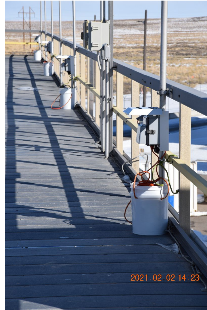
Smartphones installed on the cooling tower deck
