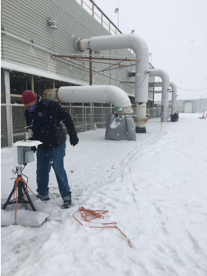
Installing smartphones near the cooling tower
