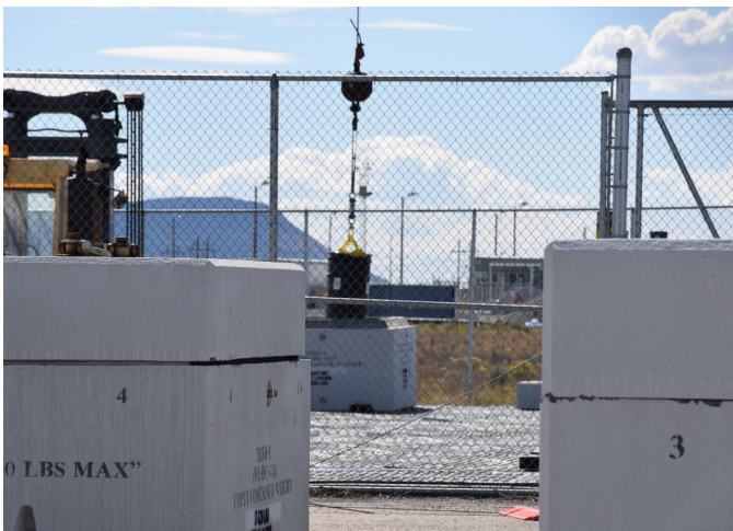
Fig 7. Placement of a 50-gallon drum with radioactive waste into the fourth position of the ISC.
