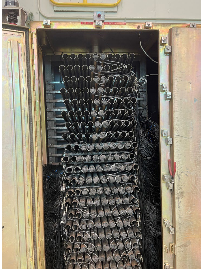
Figure 23. Photograph of the new installed detectors connected to their respective cables.
