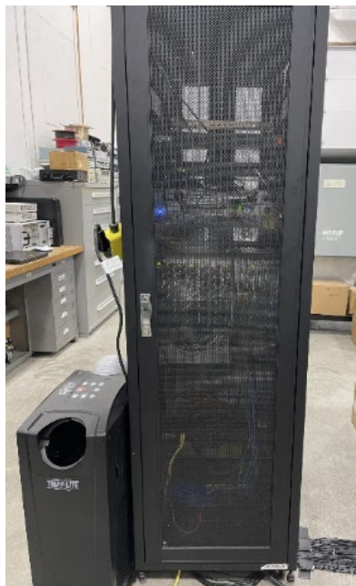
Figure 3. TRIPP-LITE cooler, shown on the left side, installed into the DAQ cabinet.
