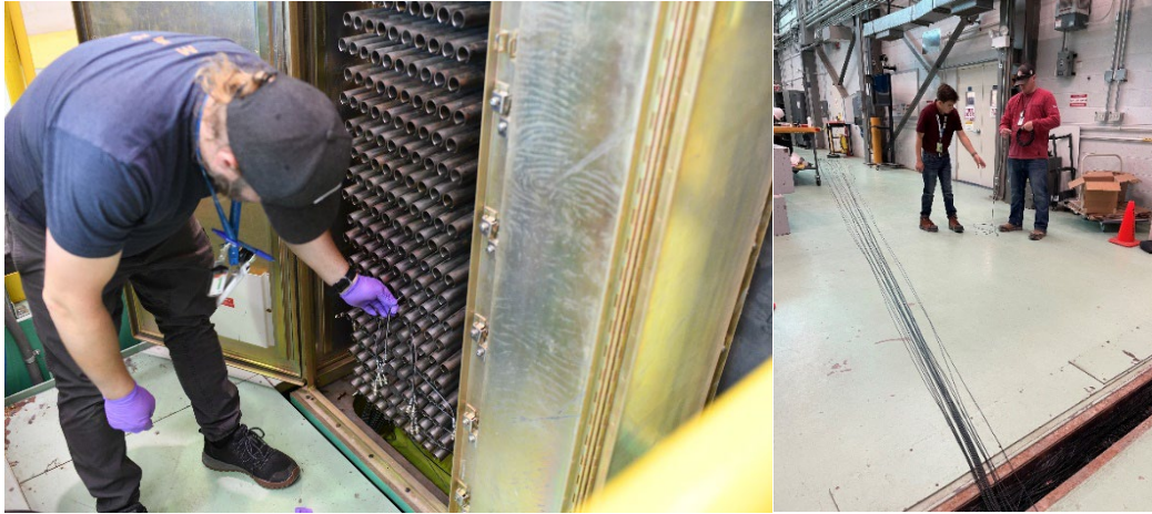
Figure 18. Disconnecting of the cables and removal of the detectors (left). Placement of the new 100-foot cables (right).
