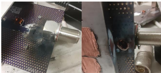
Figure 5. Damage caused by arcing on new damper filters
