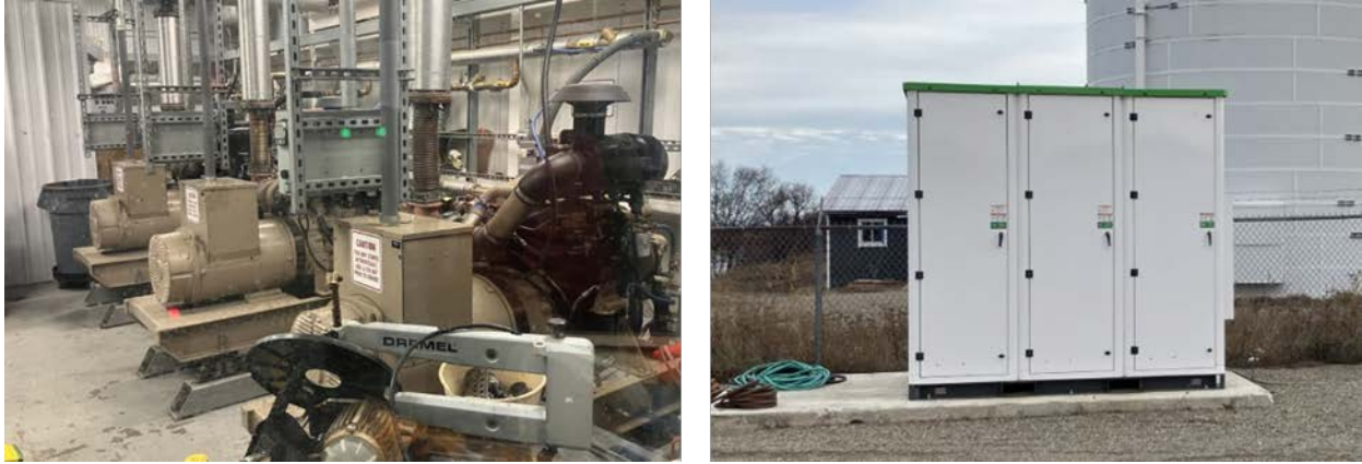
Figure 3. (left) Diesel power plant and (right) battery energy storage system in Igiugig.
