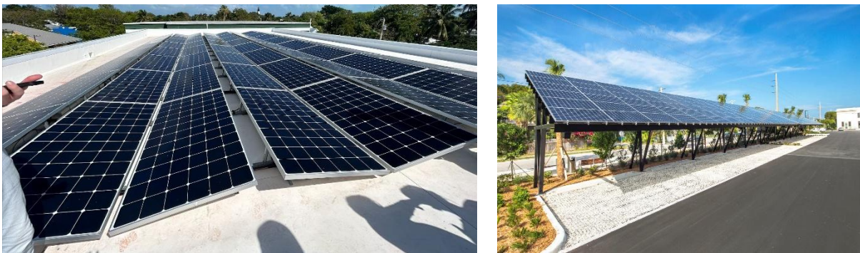
Figure 8. PV panels installed in the Frederick Douglass Community Center (left) and Glynn Archer City Hall (right)
