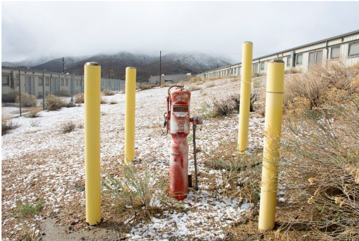
DRI Photo: DSC_4668. AR1 Fire Protection System Upright. Elevation: N/A Direction facing: South Photographer: DRI Date: March 23, 2020
