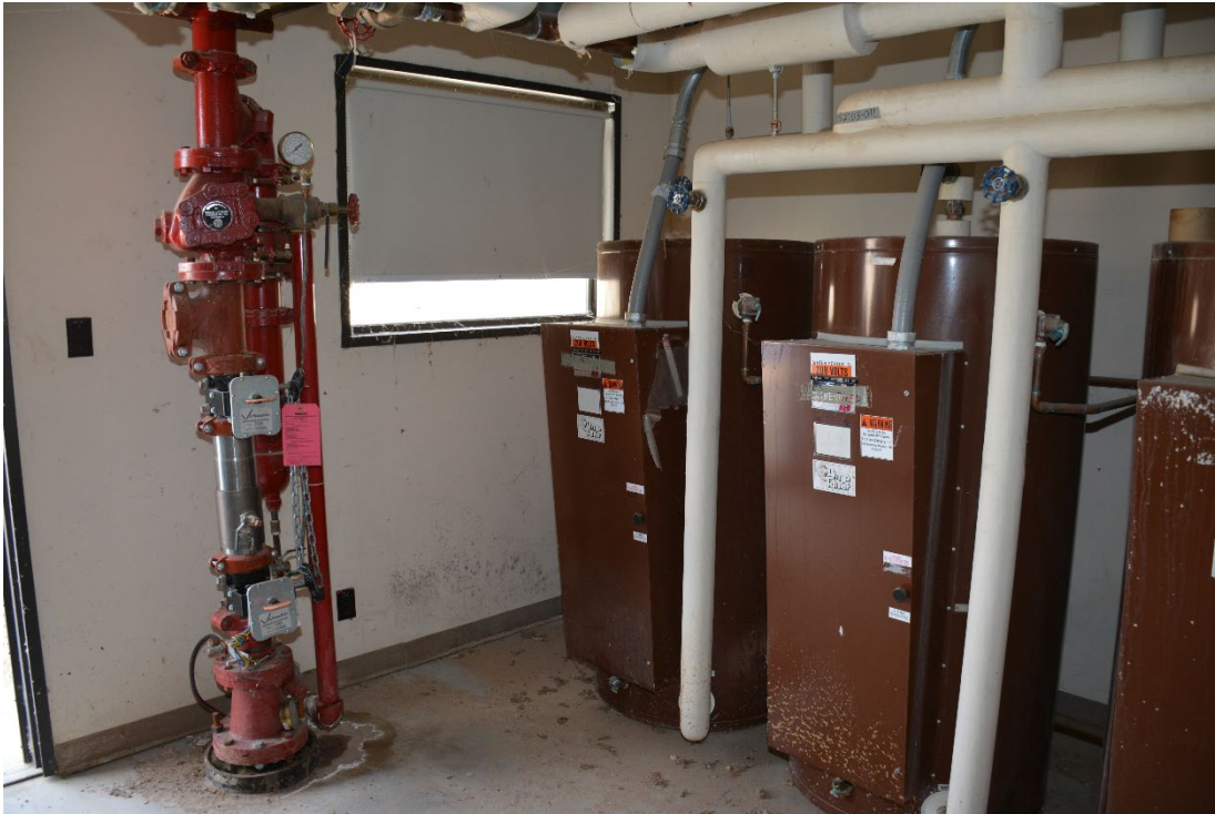
DRI Photo 11: 2531_1618. Room 48, mechanical/equipment room interior, hot water heaters and water main. Elevation: NA Direction facing: Northwest Photographer: DRI Date: April 17, 2025
