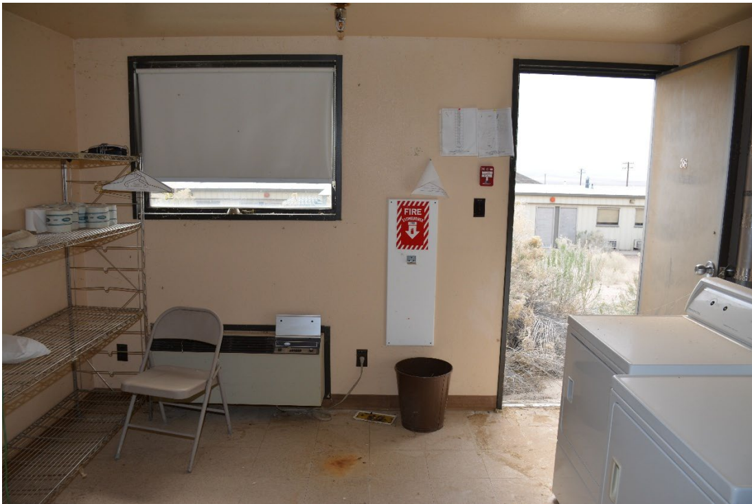
DRI Photo 19: 2531_1574. Room 36, public laundry room interior, dryers, air-conditioner, and wire shelving. Elevation: NA Direction facing: East Photographer: DRI Date: April 17, 2025
