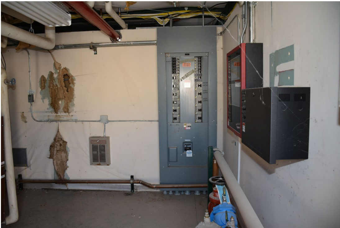
DRI Photo 10: 2531_1617. Room 48, mechanical/equipment room interior, breaker box. Elevation: NA Direction facing: East Photographer: DRI Date: April 17, 2025
