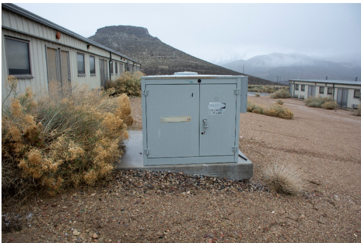
DRI Photo: DSC_4636. AR2 Transformer.
