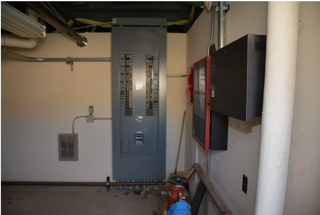
DRI Photo 15: 2531_1610. Room 13, mechanical/equipment room interior, breaker box. Elevation: NA Direction facing: East Photographer: DRI Date: April 17, 2025
