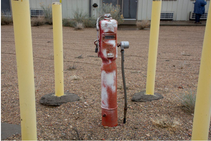
DRI Photo: DSC_4749. AR3 Fire Protection System Upright. Elevation: N/A Direction facing: East Photographer: DRI Date: March 23, 2020
