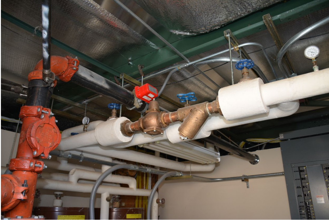
DRI Photo 14: 2531_1609. Room 13, mechanical/equipment room interior, ceiling detail. Elevation: NA Direction facing: Detail Photographer: DRI Date: April 17, 2025
