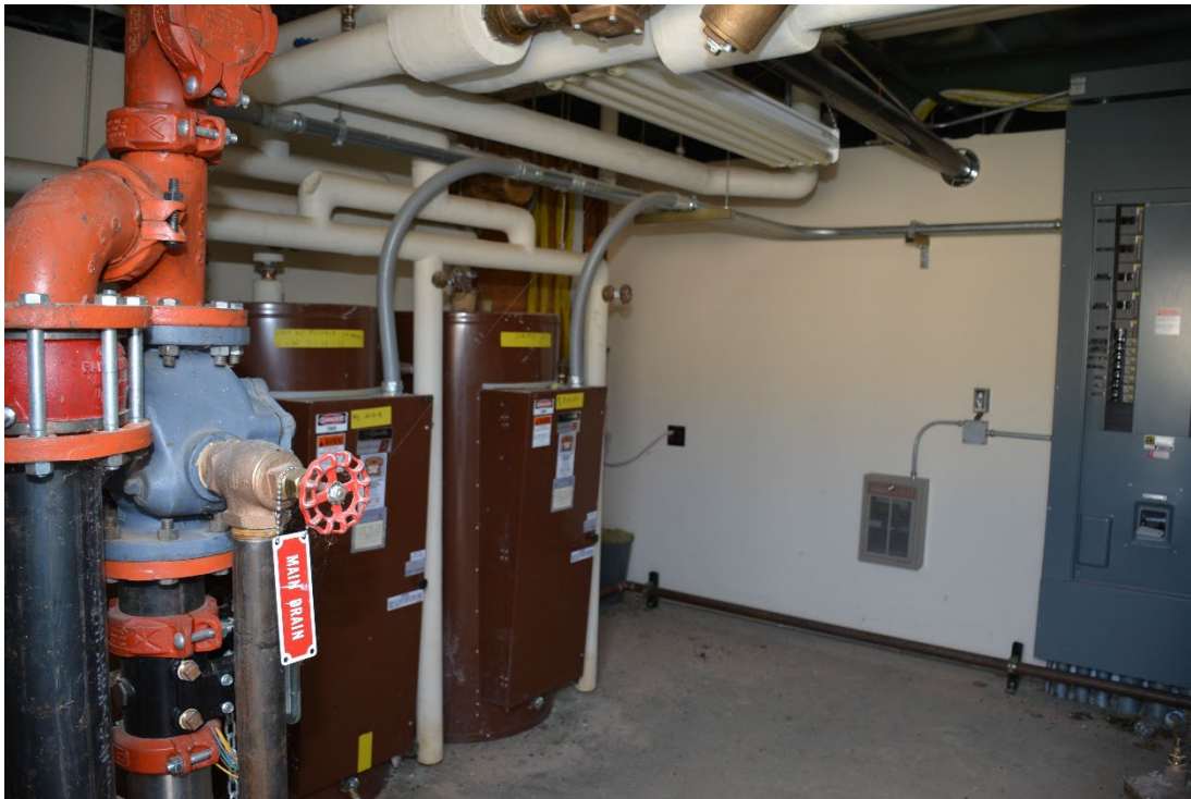
DRI Photo 13: 2531_1608. Room 13, mechanical/equipment room interior, hot water heaters, breaker box, water main. Elevation: NA Direction facing: Northeast Photographer: DRI Date: April 17, 2025
