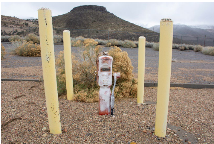
DRI Photo: DSC_4668. AR2 Fire Protection System Upright. Elevation: N/A Direction facing: North Photographer: DRI Date: March 23, 2020
