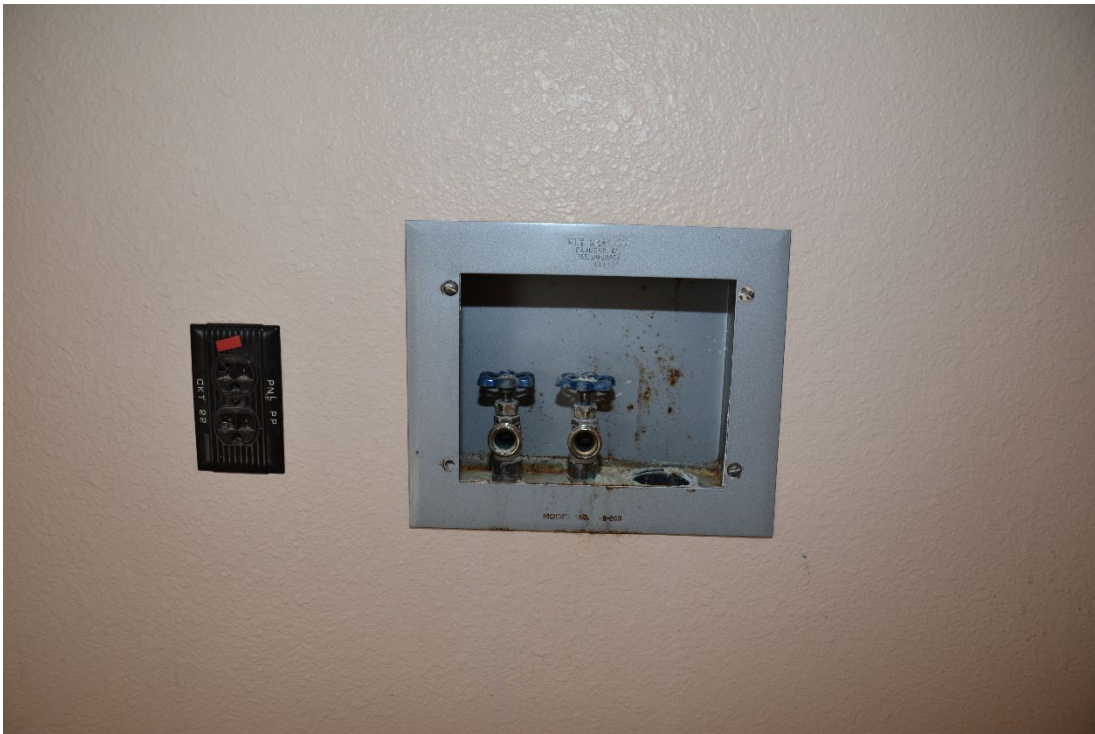
DRI Photo 9: 2531_1590. Room 47, public laundry room, water valve detail, west wall. Elevation: NA Direction facing: Detail Photographer: DRI Date: April 17, 2025
