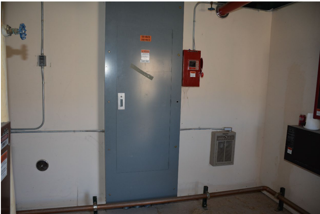
DRI Photo 11: 2531_1621. Room 48, mechanical/equipment room interior, breaker box and wall heater.
