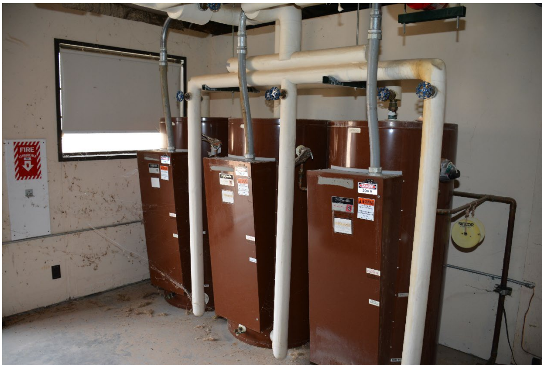
DRI Photo 13: 2531_1623. Room 48, mechanical/equipment room interior, hot water heaters. Elevation: NA Direction facing: Northwest Photographer: DRI Date: April 17, 2025
