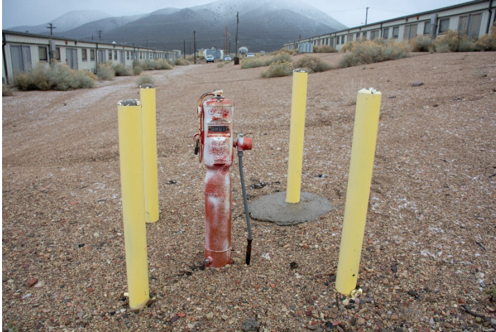
DRI Photo: DSC_4620. AR3 Fire Protection System Upright. Elevation: N/A Direction facing: South Photographer: DRI Date: March 23, 2020
