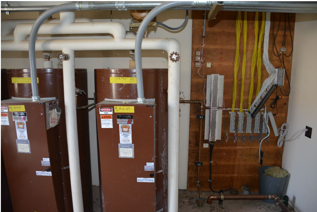
DRI Photo 17: 2531_1612. Room 13, mechanical/equipment room interior, hot water heaters, and phone panel. Elevation: NA Direction facing: North Photographer: DRI Date: April 17, 2025
