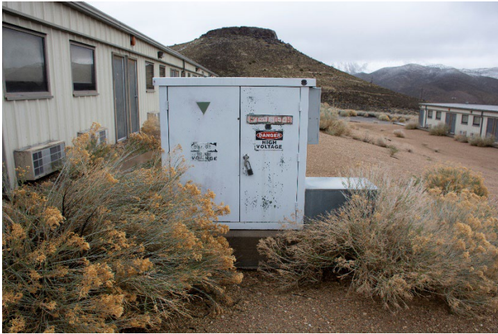
DRI Photo: DSC_4732. AR1 Transformer. Elevation: N/A Direction facing: North Photographer: DRI Date: March 23, 2020
