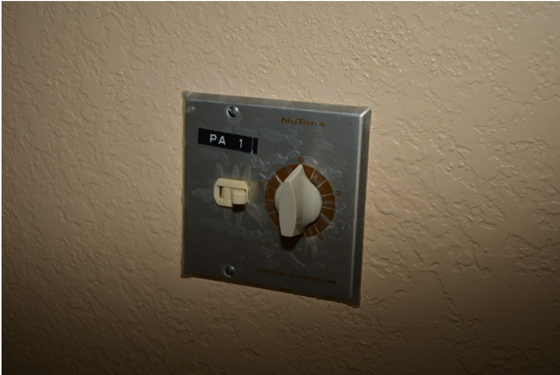
DRI Photo 9: 2531_1560. Room 1, ADA-accessible bathroom, heater lamp switch. Elevation: NA Direction facing: Detail Photographer: DRI Date: April 17, 2025
