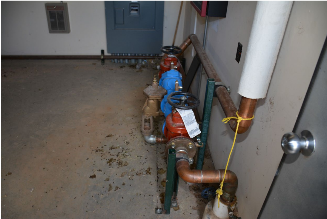
DRI Photo 16: 2531_1611. Room 13, mechanical/equipment room interior, fire control valve detail. Elevation: NA Direction facing: Detail Photographer: DRI Date: April 17, 2025
