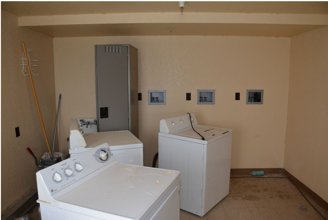
DRI Photo 11: 2531_1576. Room 36, public laundry room interior. Elevation: NA Direction facing: West Photographer: DRI Date: April 17, 2025
