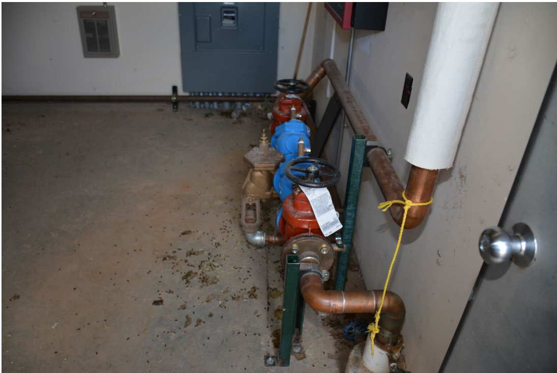
DRI Photo 21: 2531_1611. Room 13, mechanical/equipment room interior, fire control valve. Elevation: NA Direction facing: Detail Photographer: DRI Date: April 17, 2025
