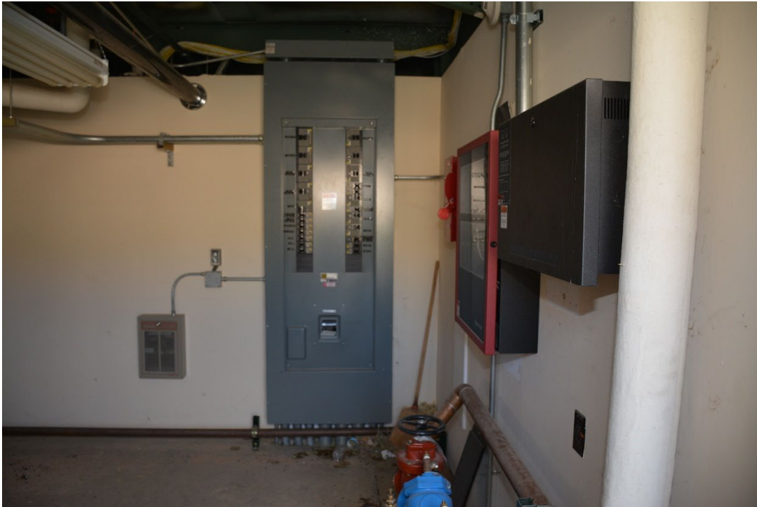
DRI Photo 20: 2531_1610. Room 13, mechanical/equipment room interior, breaker box. Elevation: NA Direction facing: East Photographer: DRI Date: April 17, 2025
