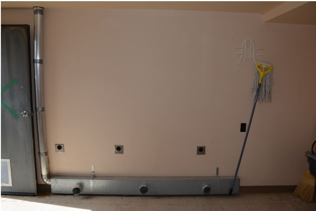
DRI Photo 8: 2531_1583. Room 47, public laundry room, dryer vent detail. Elevation: NA Direction facing: South Photographer: DRI Date: April 17, 2025
