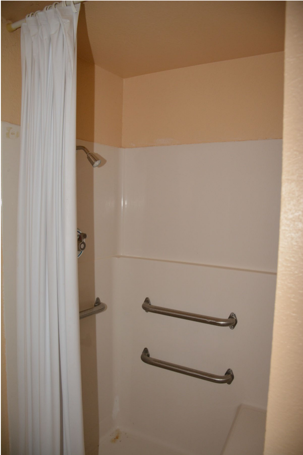
DRI Photo 7: 2531_1558. Room 1, ADA-accessible bathroom, shower interior. Elevation: NA Direction facing: Detail Photographer: DRI Date: April 17, 2025
