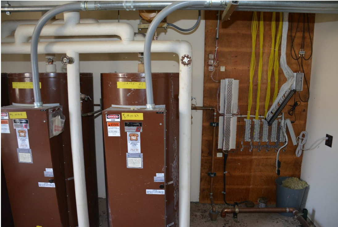
DRI Photo 22: 2531_1612. Room 13, mechanical/equipment room interior, water heaters and electrical panel. Elevation: NA Direction facing: North Photographer: DRI Date: April 17, 2025
