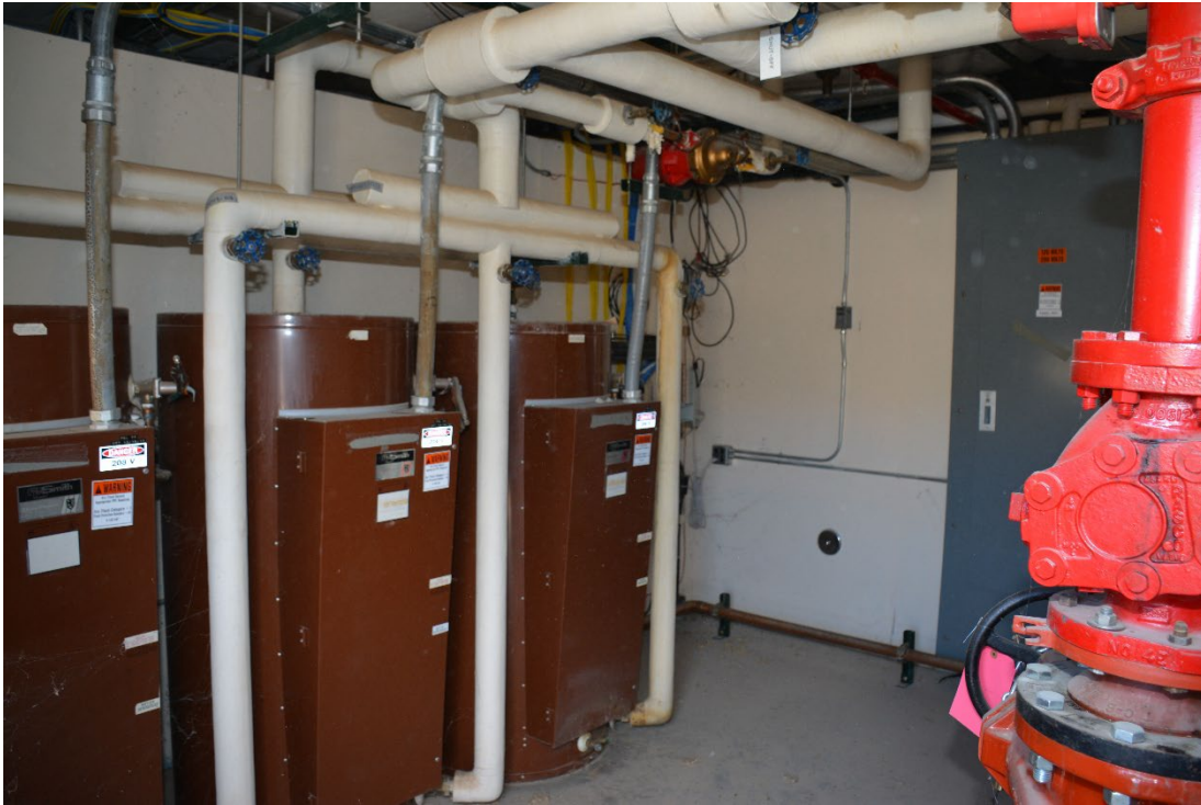
DRI Photo 10: 2531_1620. Room 48, mechanical/equipment room interior, hot water heaters, breaker box, and water main.
