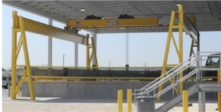
Figure 5-5. Free Standing Bridge Crane
