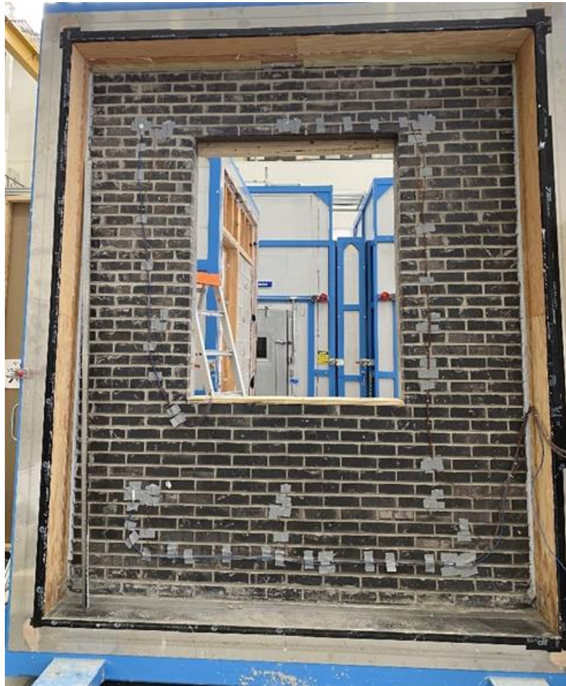
Figure 3. Wall representing "existing" masonry wall with one CMU layer and a brick layer: before installation of the hydronic shell
