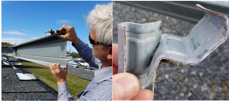
Figure 2. Inadequate frame stiffness and fastener strength led to failures
