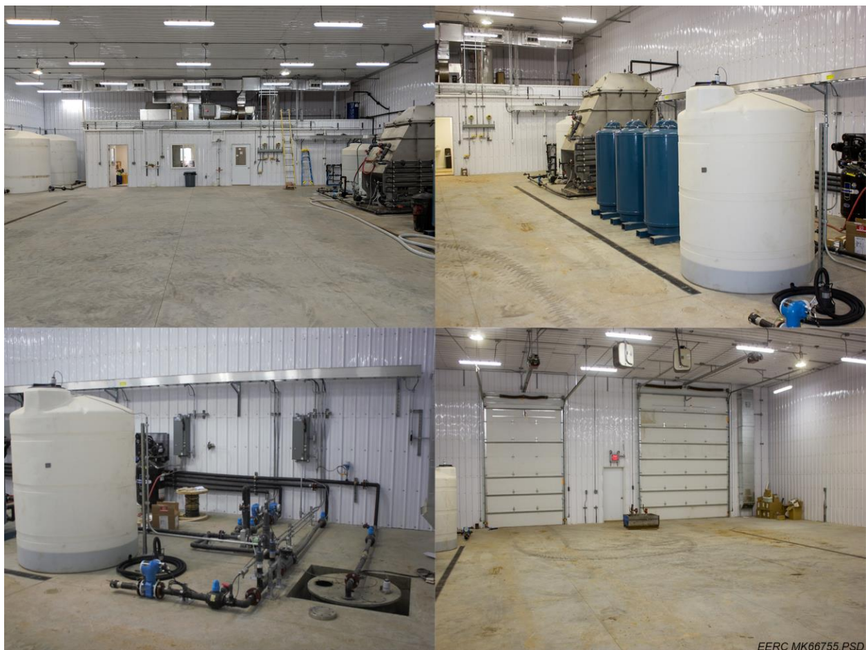
Figure 7. Various photos and angles of the treatment facility.
