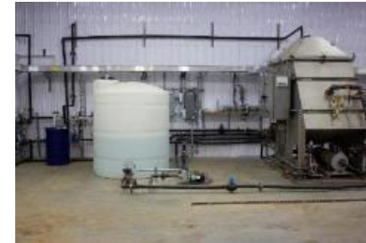
Water Blending and Pretreatment
