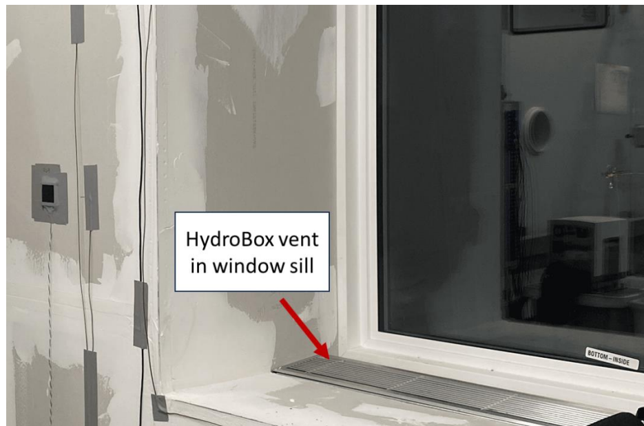
Figure 3. Vent in the window-sill from where the fan in the HydroBox blows conditioned air to space
