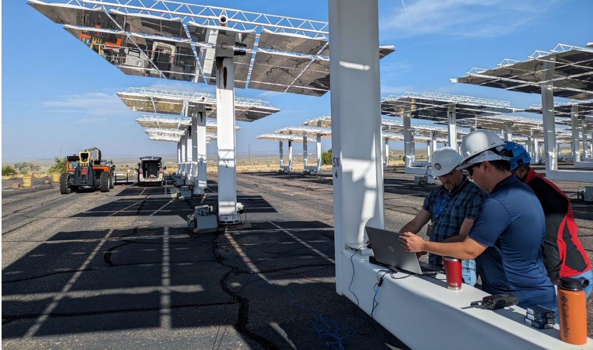
Figure 57. Initial Field-Testing Using Heliostat 05W06.
