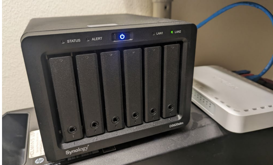
Figure 48. Installed network attached storage (NAS).
