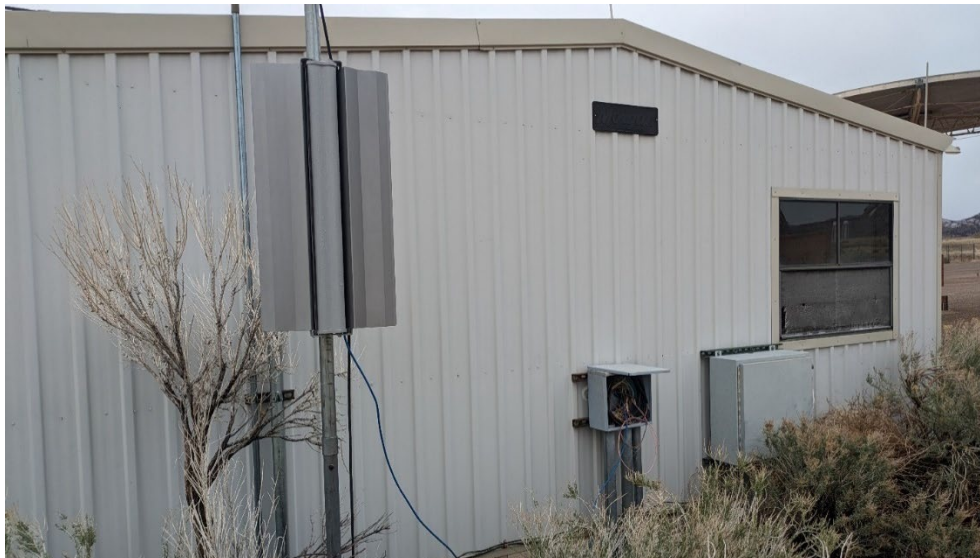
Figure 25. Communications Station Antenna.
