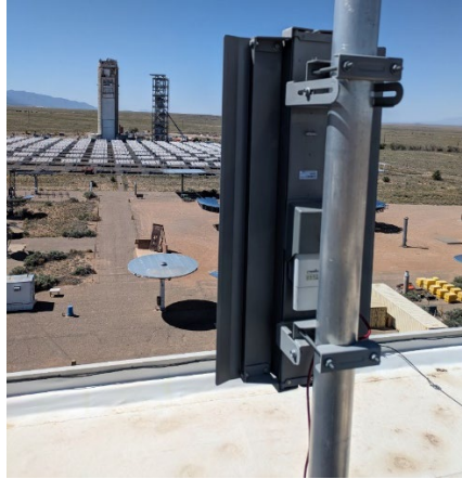
Figure 36. Control Room Antenna Permanent Location.
