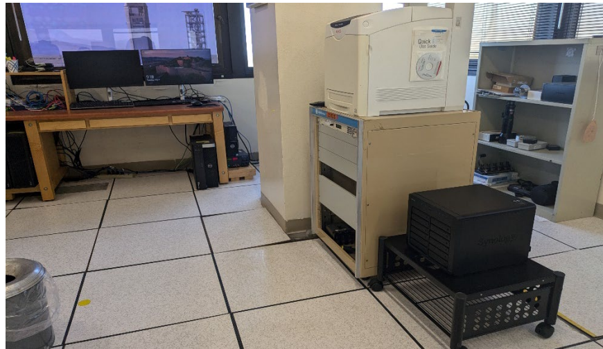
Figure 49. Permanent Installation of NAS System.
