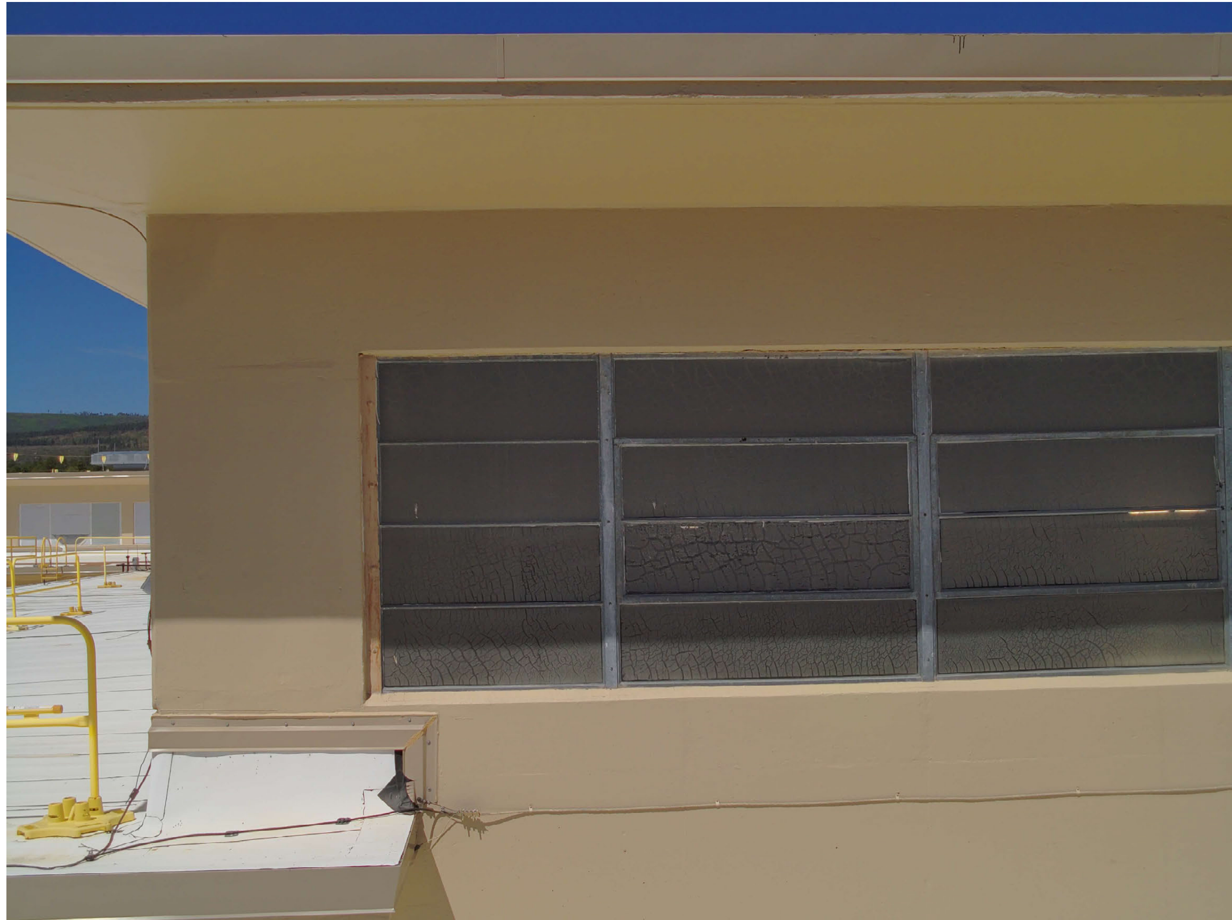
TA-03-0039 center wing, east facade, cracked window coating and delaminated glazing detail
