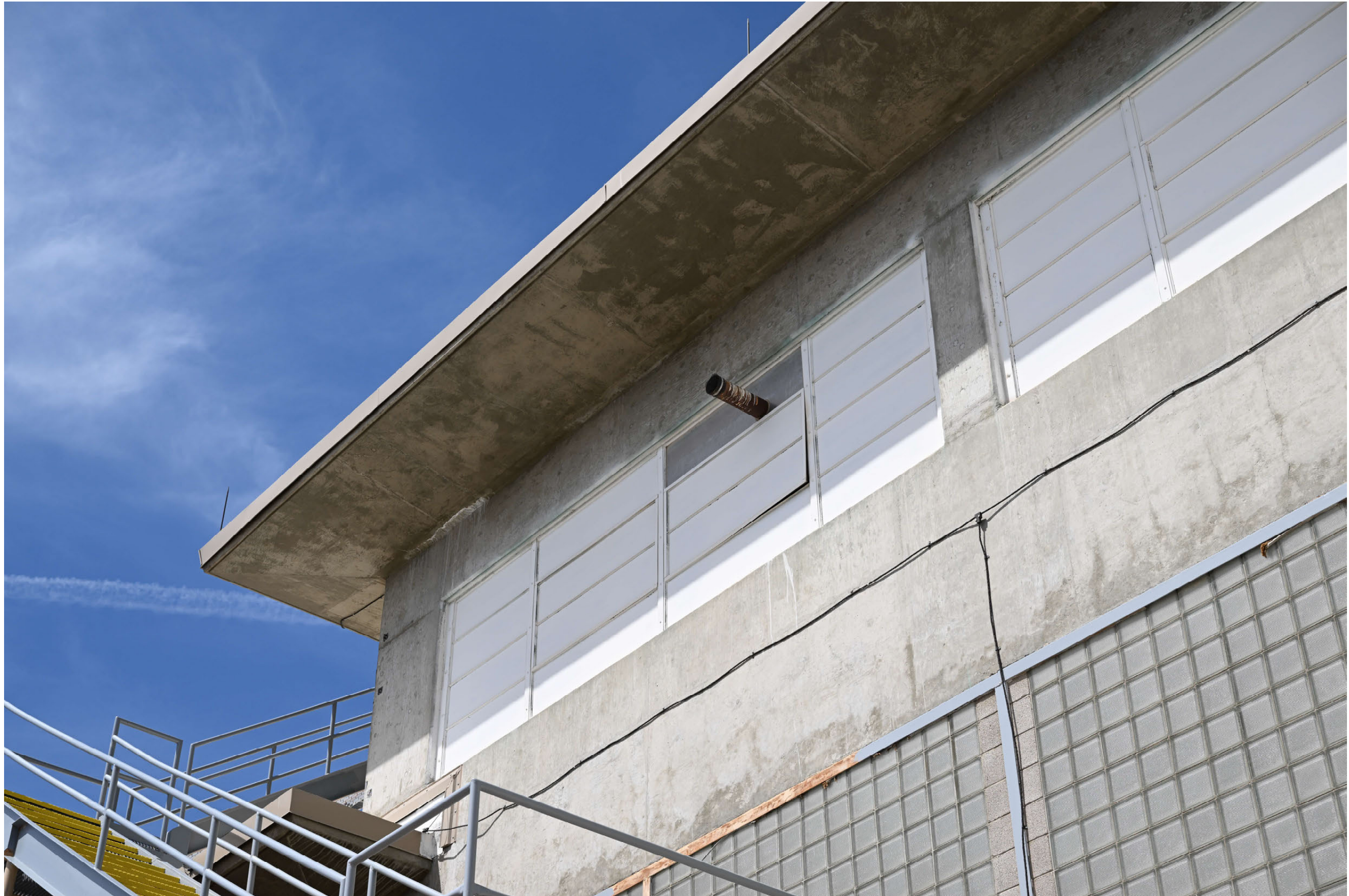
TA-03-0039 south wing, east facade vent penetration and sash damage detail
