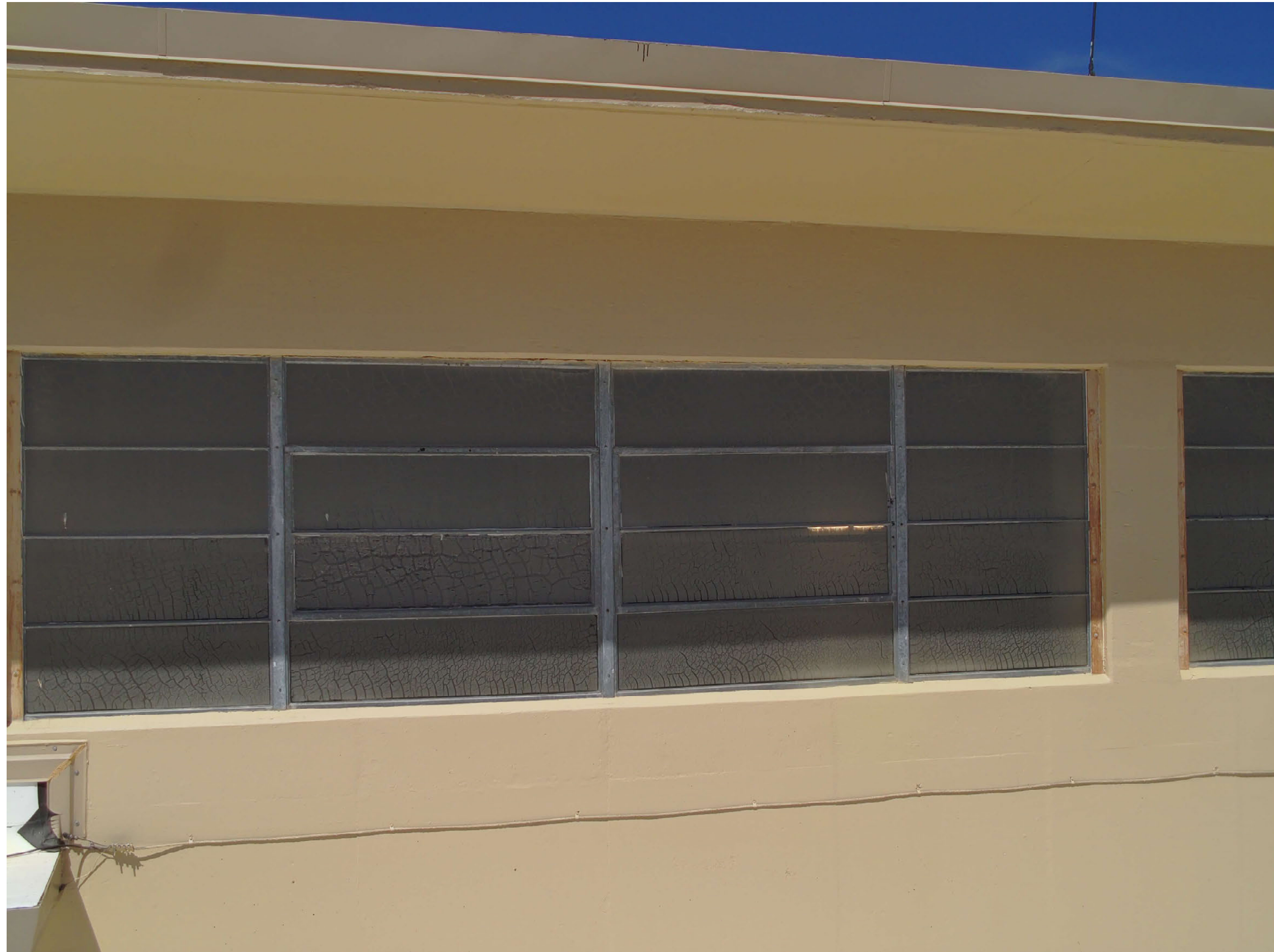
TA-03-0039 center wing, east facade, cracked window coating and delaminated glazing detail
