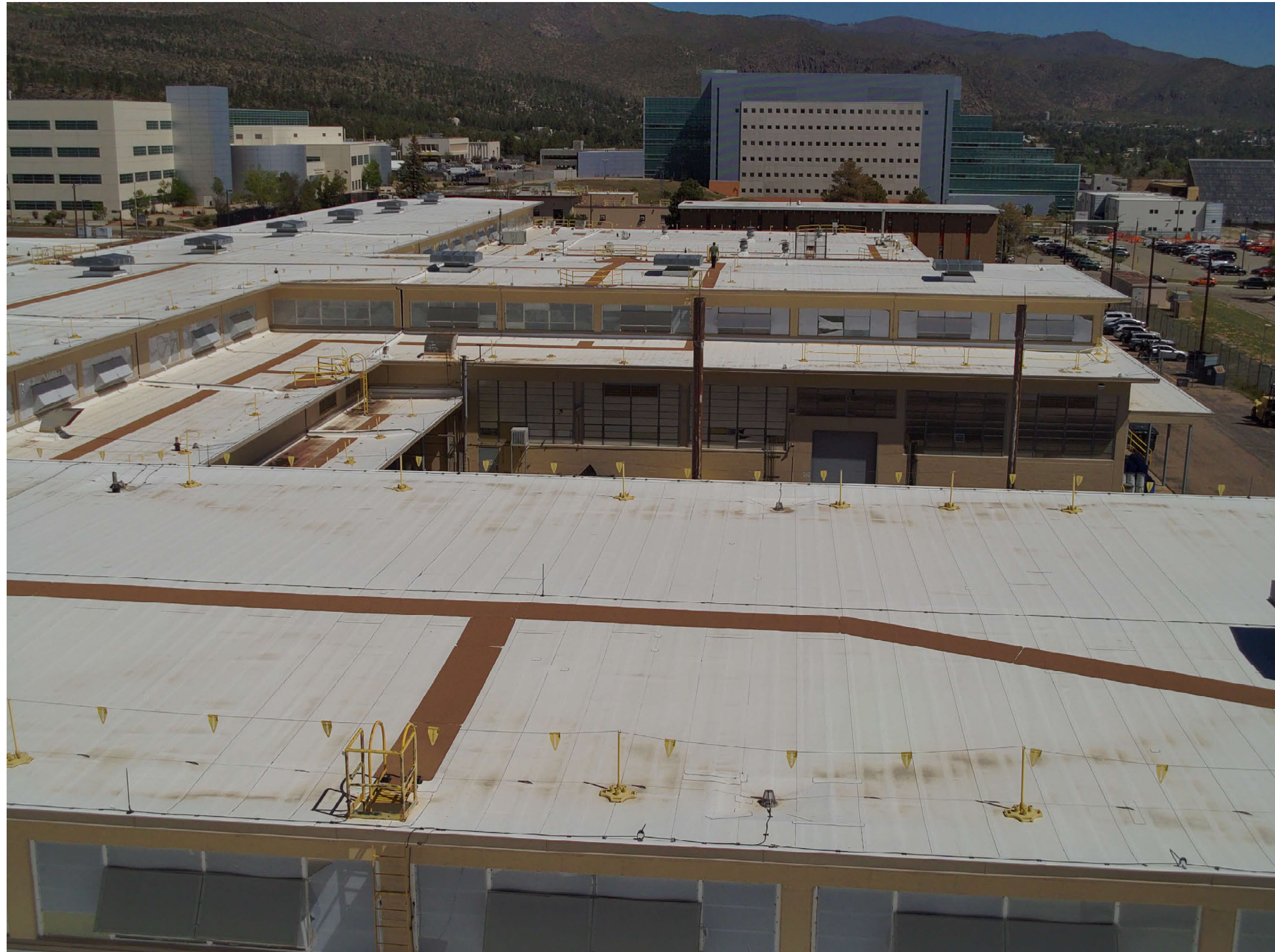
TA-03-0039 south wing (foreground), south portion of spine (left), center wing (center), north portion of spine (back left), north wing (background), south and east facades
