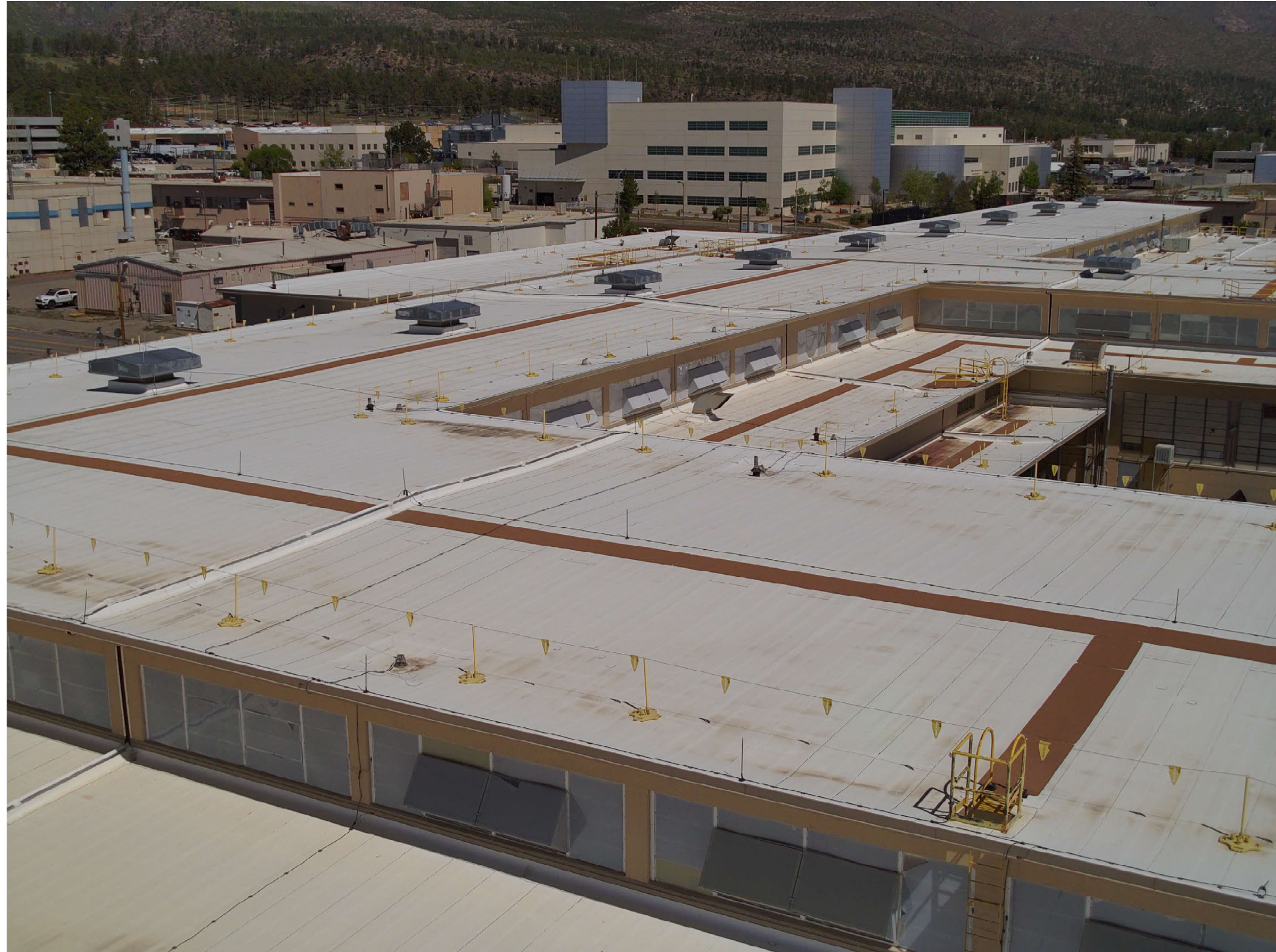
TA-03-0039 south wing (foreground), south portion of spine (center), center wing (right), north portion of spine (background, south and east facades)
