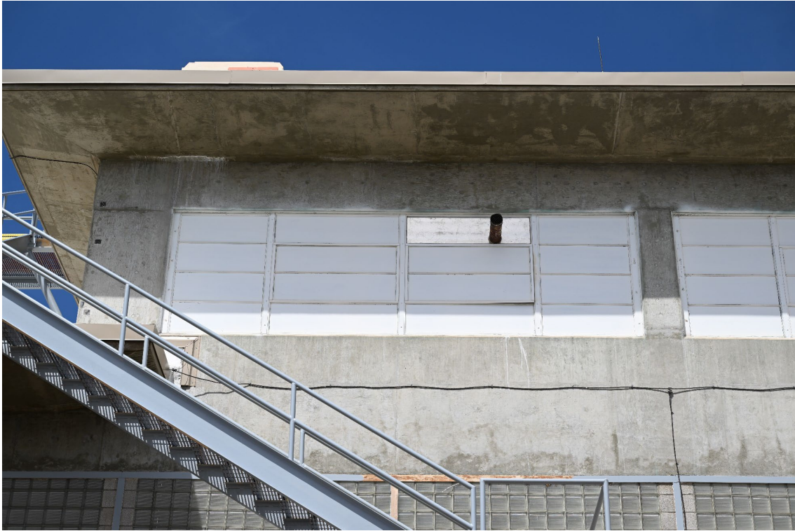
Figure 5-3. Example vent penetration, June 6, 2023 (LANL image, image no. DSC_0119).
