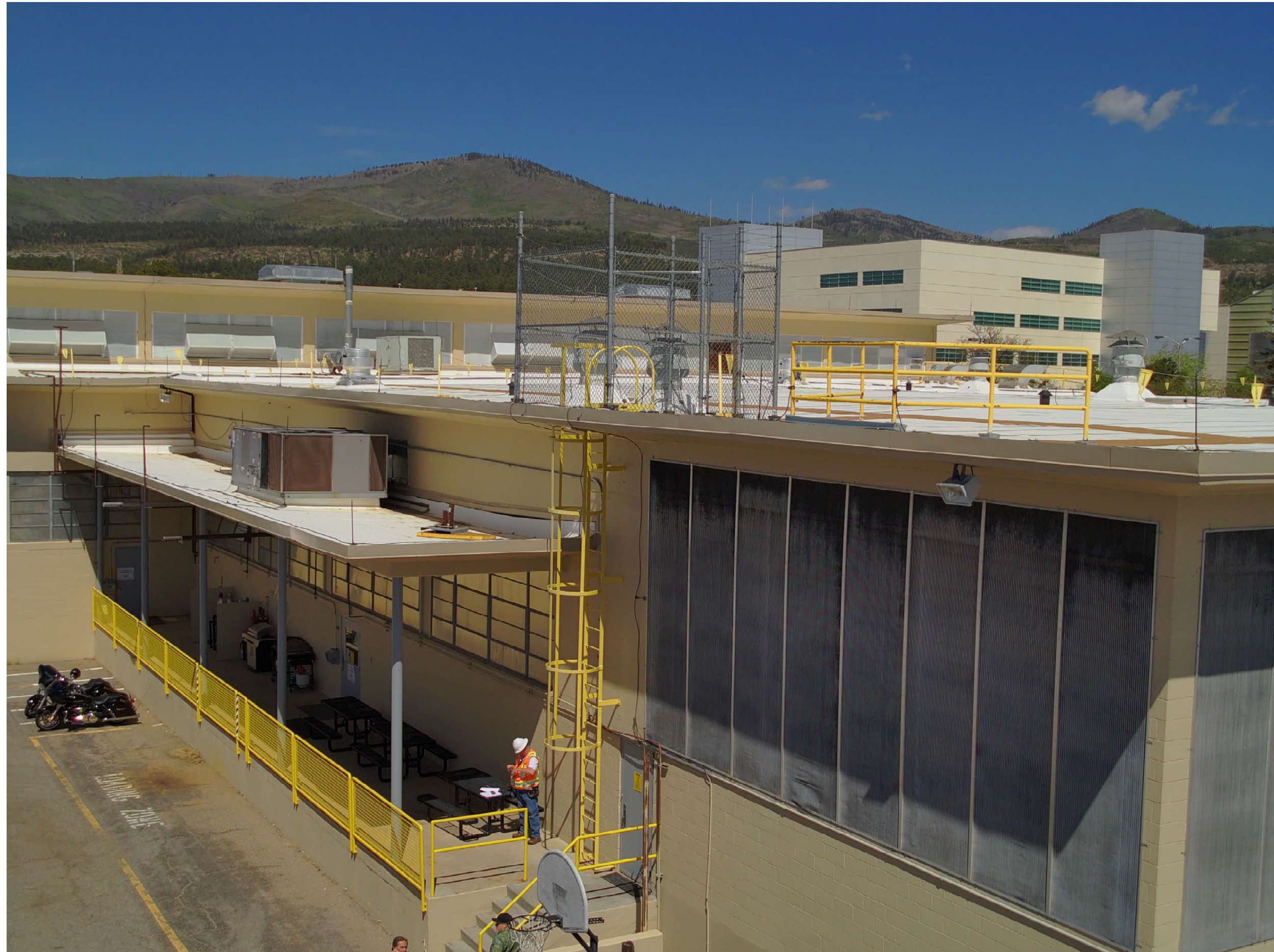
TA-03-0039 north portion of spine (left), north wing (right), east and south facades
