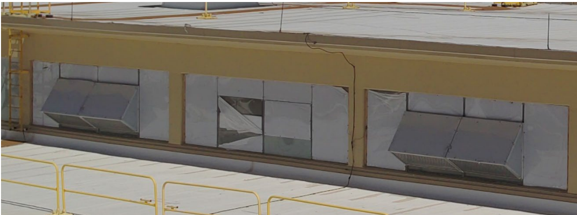
Figure 5-6. Example of broken lites with various ad hoc repairs (note center bank of windows) May 24, 2024 (LANL image, image no. S1006637).
