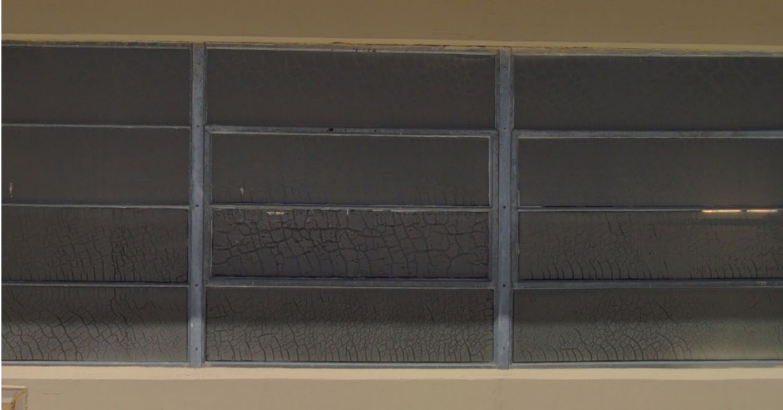
Figure 5-8. Example of delamination to window glazing and caulking, May 24, 2024 (LANL image, image no. S1006820).
