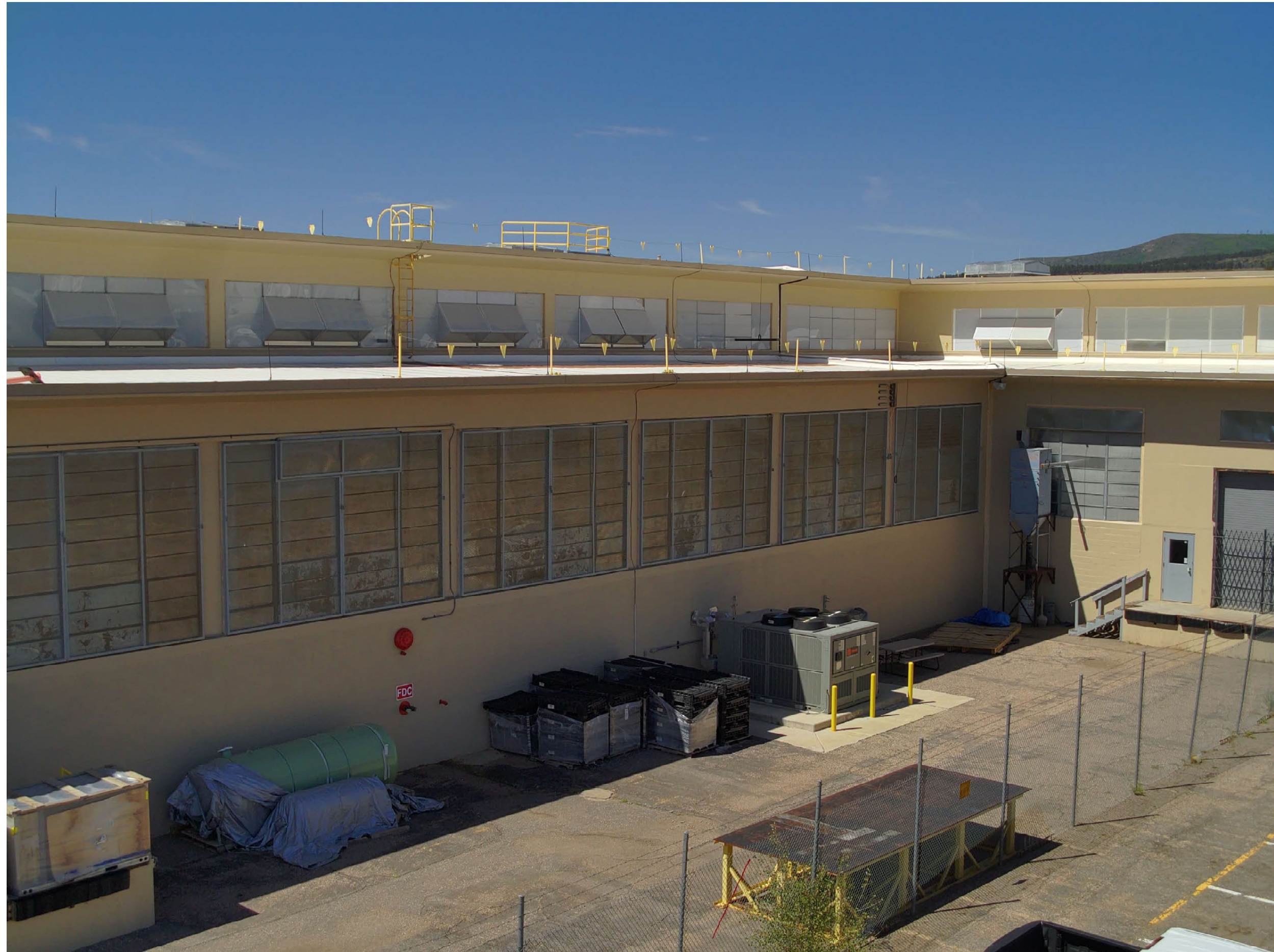
TA-03-0039 center wing (left), north portion of spine (right), north and east facades
