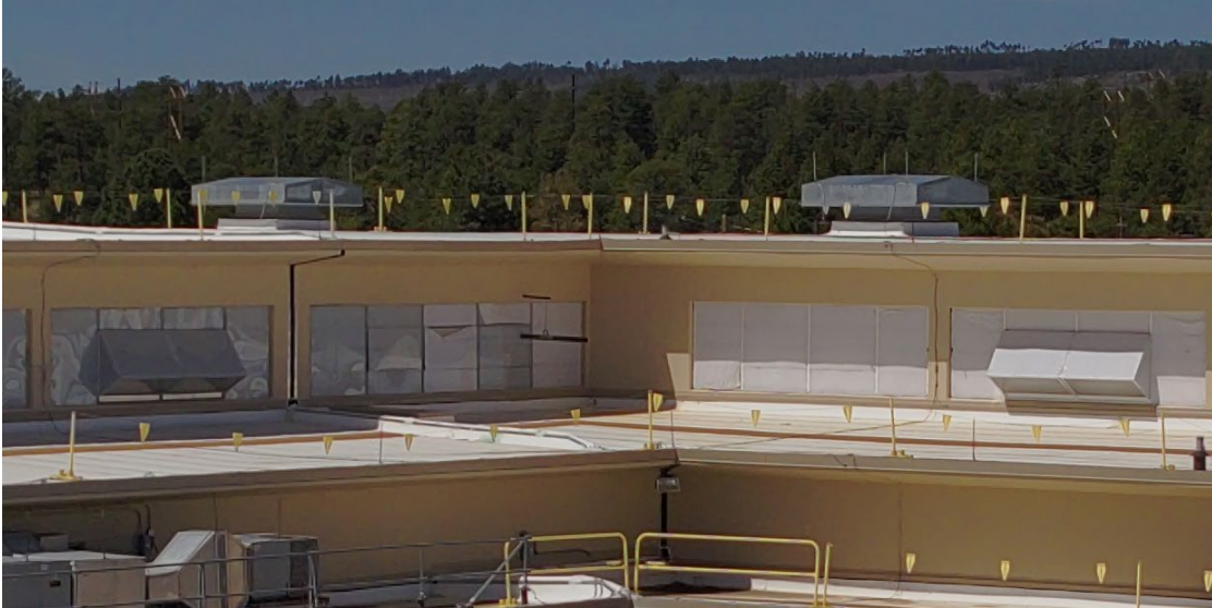
Figure 5-7. Example of broken lites with various ad hoc repairs, May 24, 2024 (LANL image, image no. S1006820).
