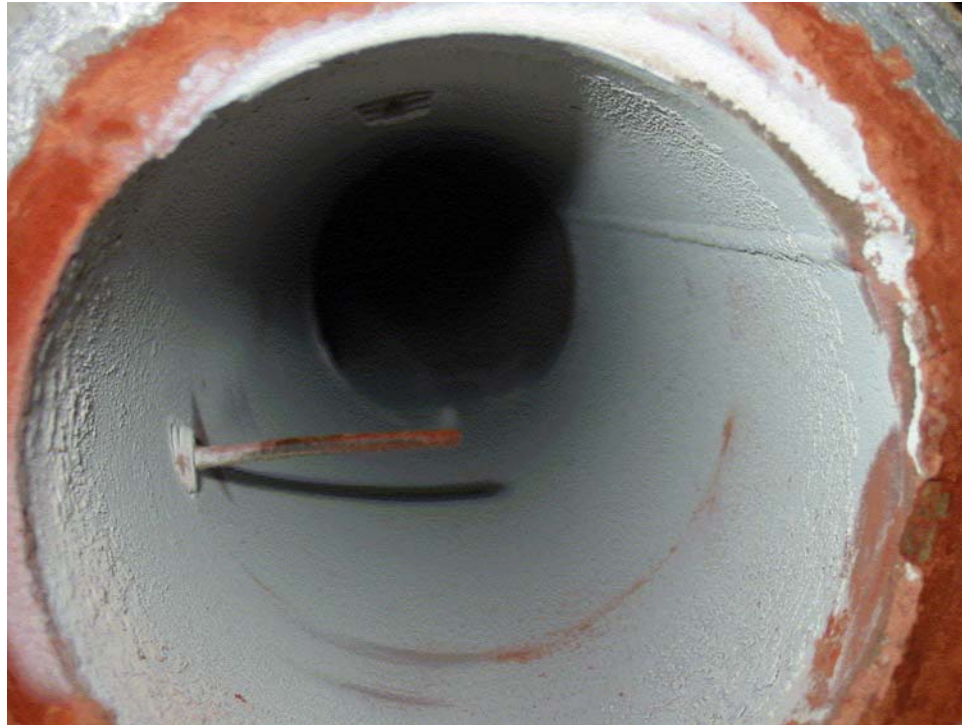
Figure 5.8. Transition line section #1 inlet.
