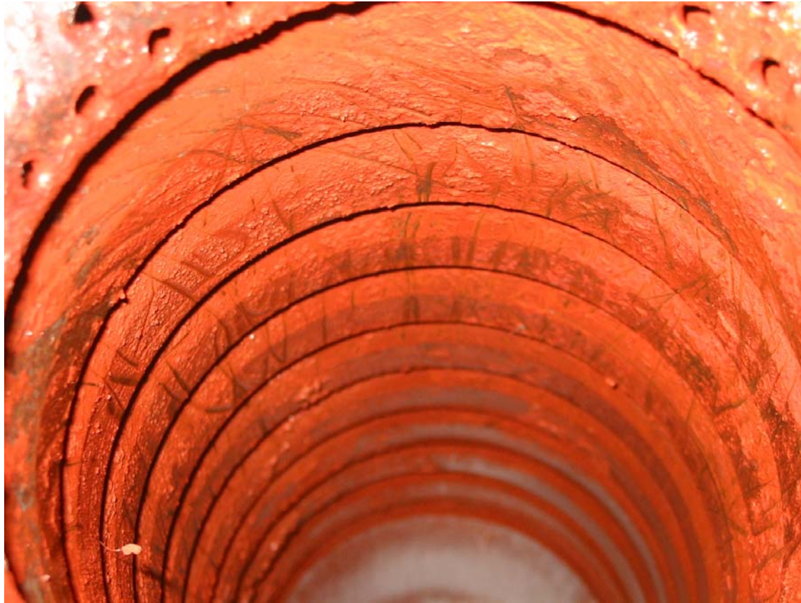
Figure 5.19. Film cooler: close-up of louvres (post cleaning).
