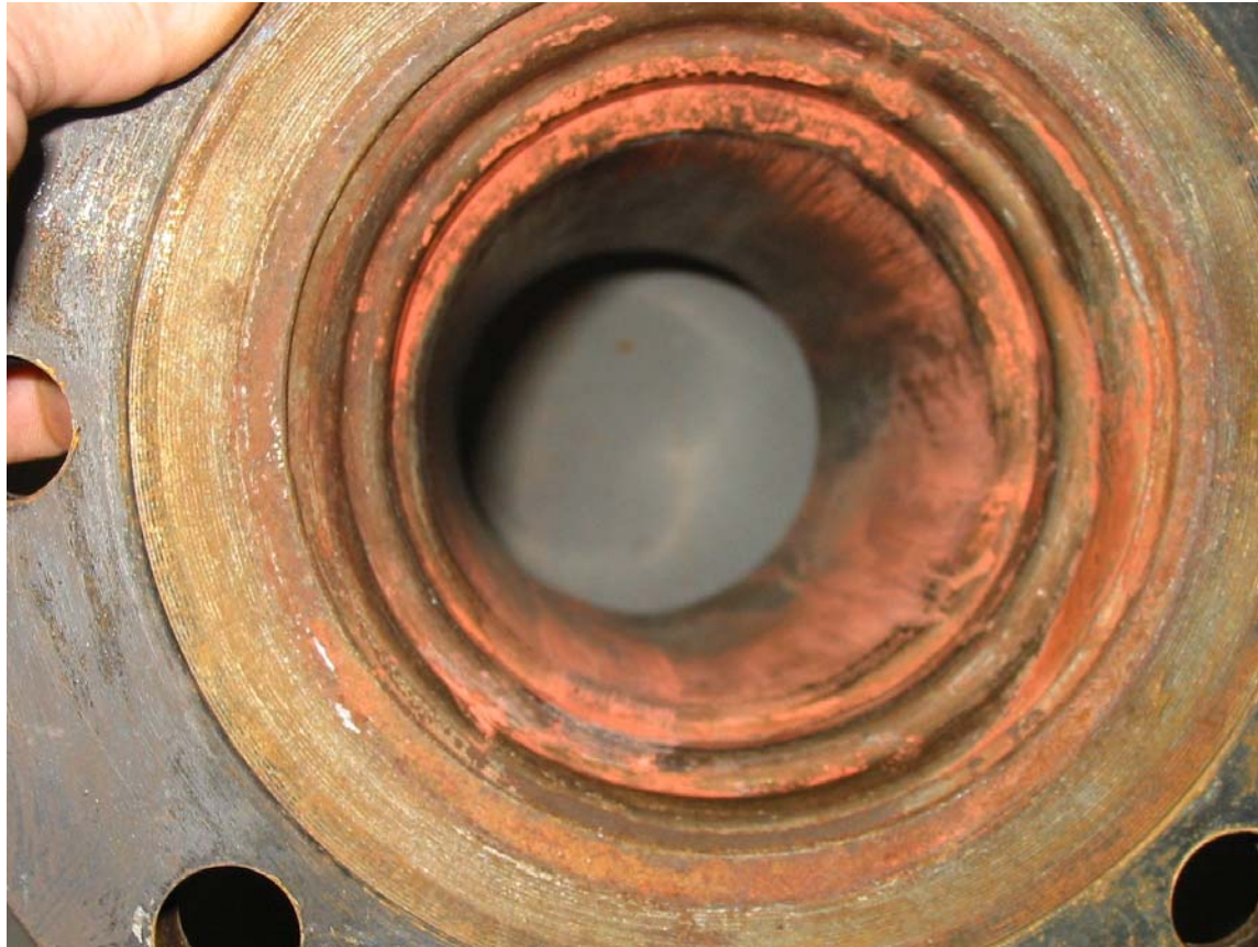
Figure 5.22. Transition line bellows inlet (post cleaning).
