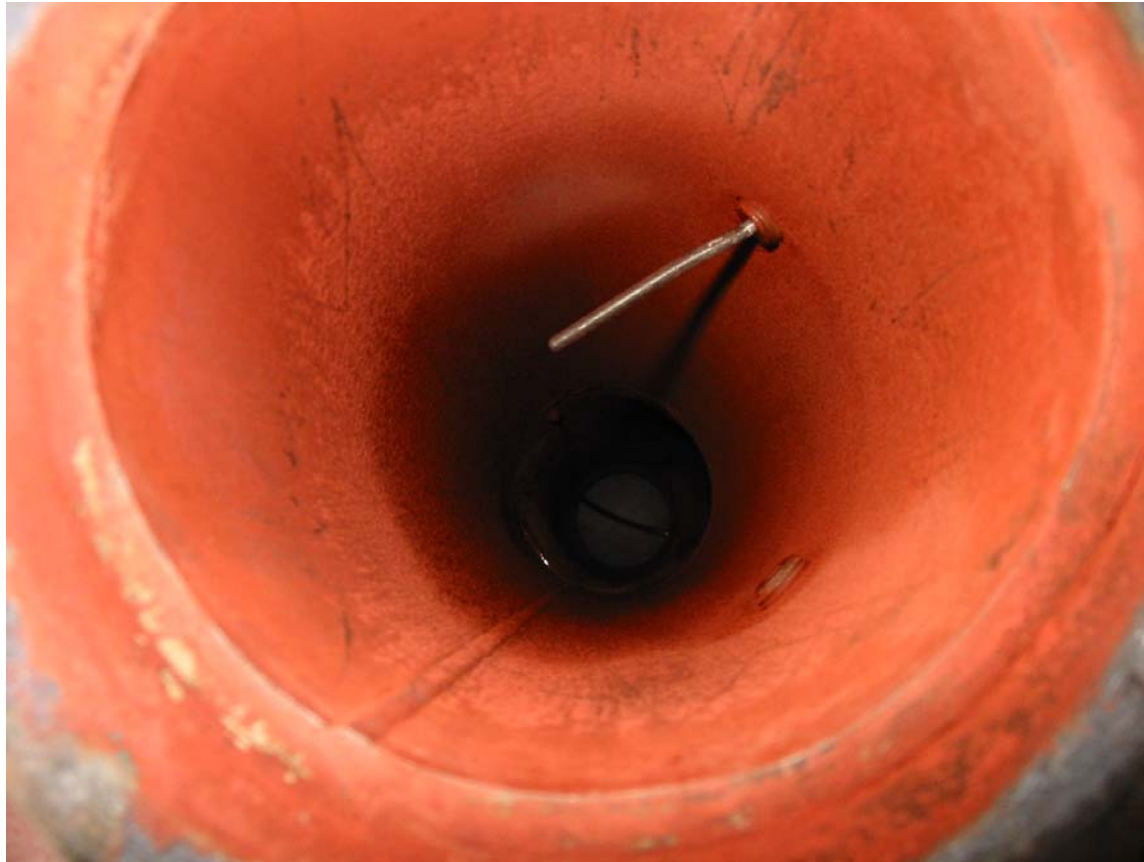
Figure 5.20. Transition line section #1 inlet-close-up (post cleaning).
