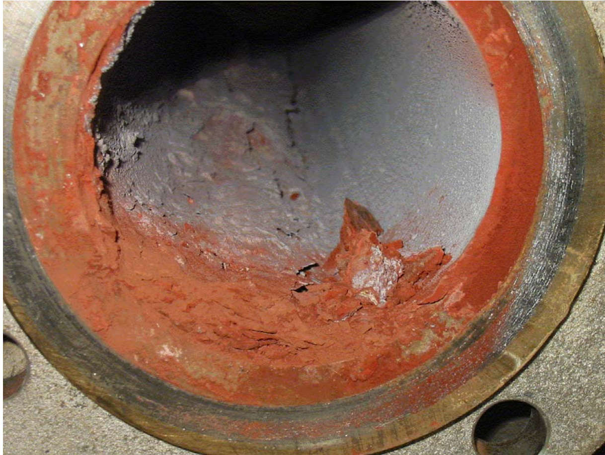
Figure 5.12. Transition line section #3 inlet.
