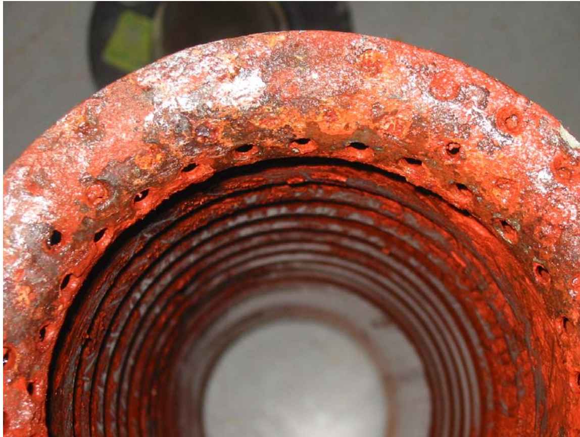
Figure 5.18. Film cooler: close-up of inlet (post cleaning).
