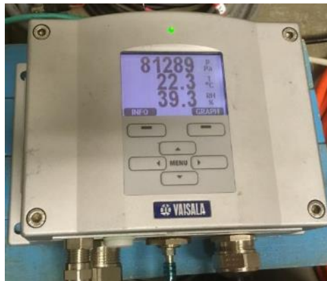
Figure 9 Vaisala Temperature Monitor within FACT Bunker
