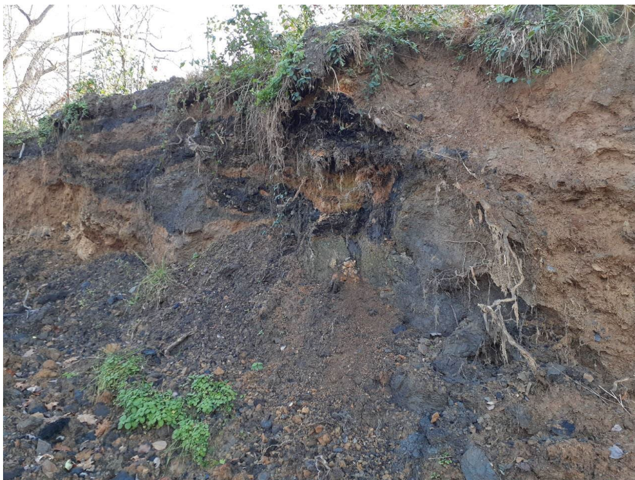
Figure 2-18. The presence of the cut into the interior slope of the mine spoil bank shows new exposure of black shales/coal fragments in the vicinity of MW-1407 & MW 1408. Photo date is November 16, 2021.
