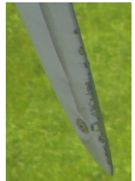
Leading edge erosion example with a conventional lightning receptor.
