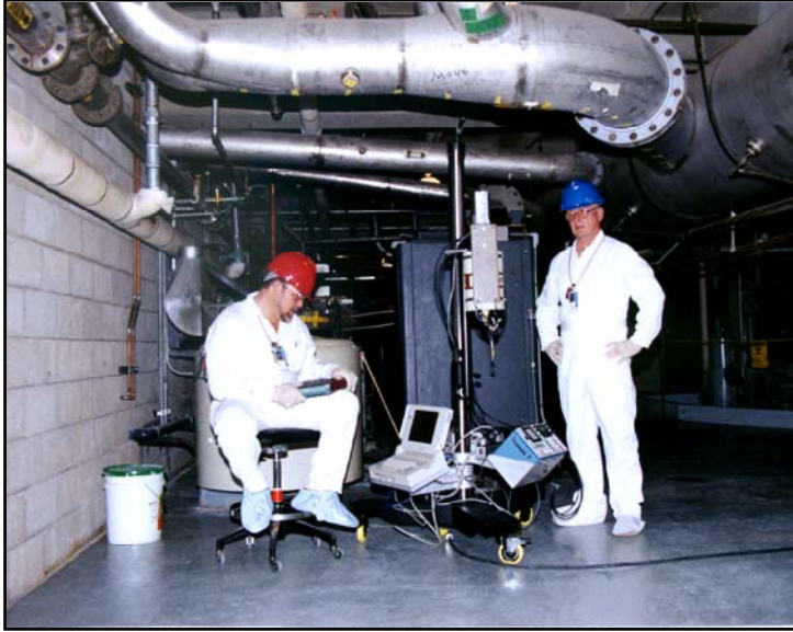
Figure VIII.5. A very large overhead duct is measured from below with a portable collimated Ge detector. The largest measurement distance for any detector positioned beneath this duct is comparable to the duct diameter because of the proximity of the equipment to the floor. The duct width is always a significant fraction of the width of the field of view of the collimated gamma-ray detector for common ventilation ducts such as this. The duct surface completely fills the field of view of this collimated detector, a geometry that is most likely (depending on the dimensions of the deposit) best-suited to analysis of the holdup as an area deposit.
