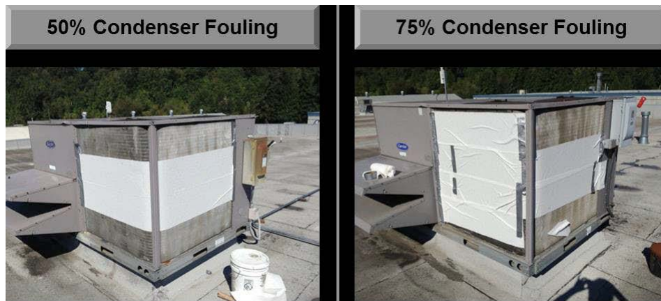
Figure 136. Condenser fouling implemented using paper
