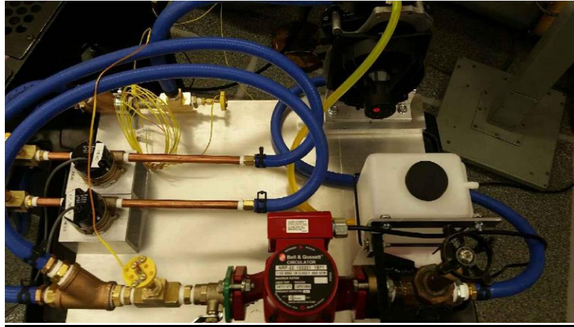
Figure 9.17. Briggs & Stratton GENSETS Cooling System Engine Operation.
