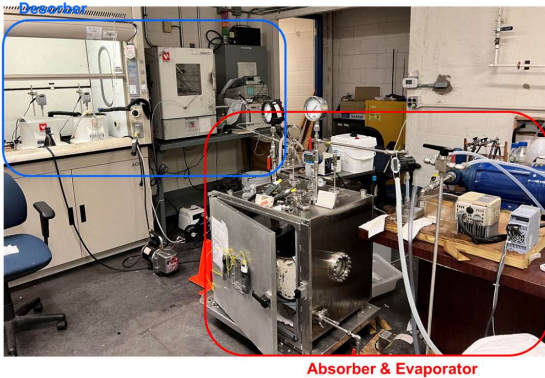
Figure 32: Picture of the prototype absorption chiller using the microemulsion as absorbent. It consists of three major components: desorber, absorber and evaporator.
